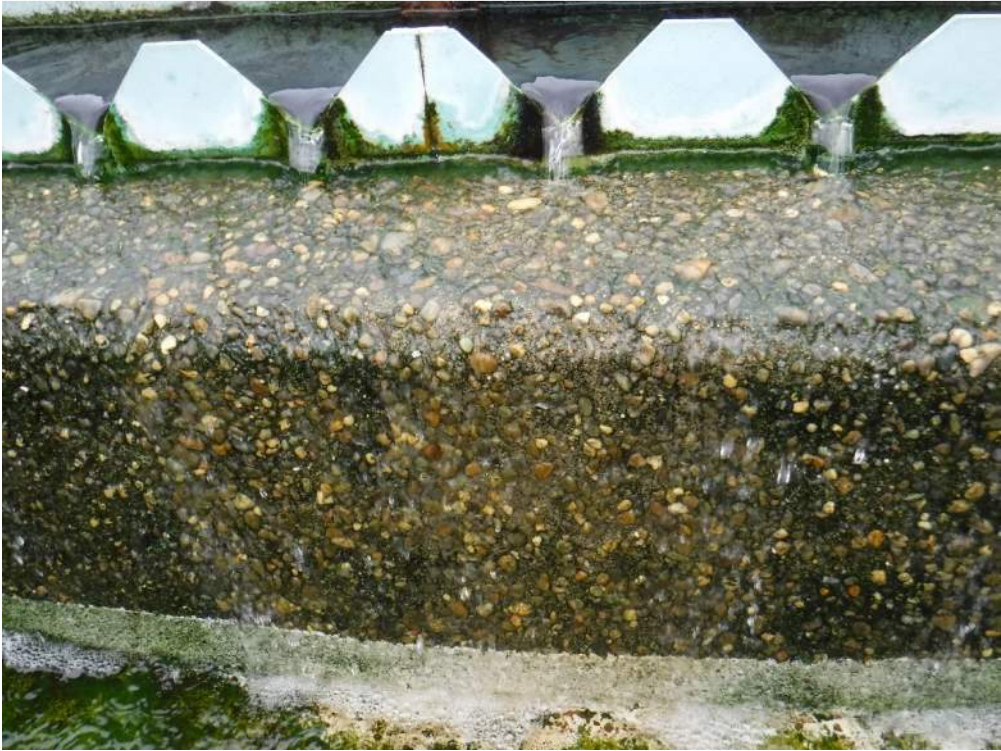
Photo 46. Exposed aggregate in launder, north secondary clarifier.
