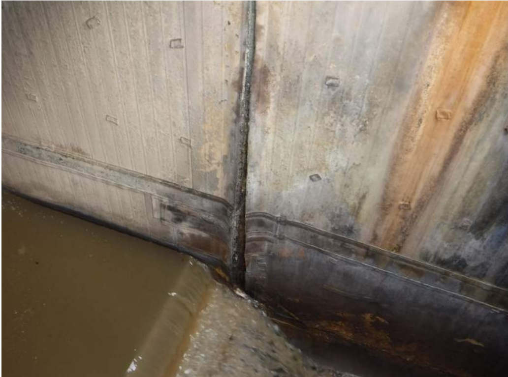
Photo 38. Embedded liner pulling from concrete at temporary gate groove, RAS return basin.
