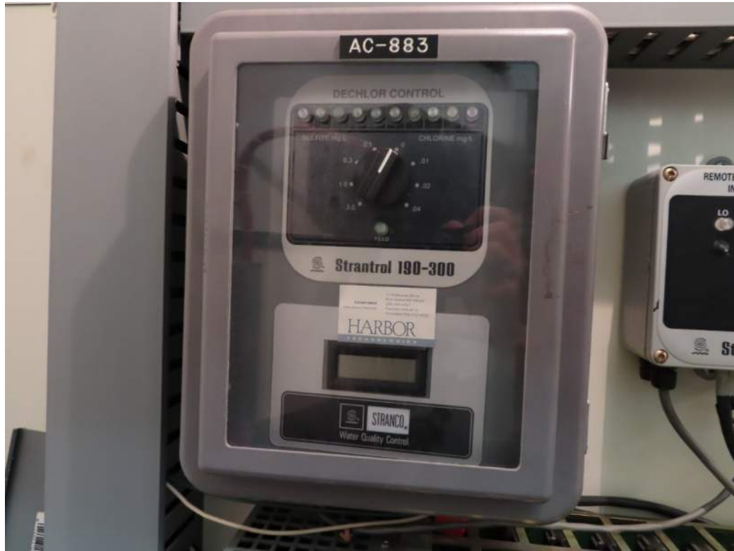
Photo 33. Deenergized Strantrol Dechlor controller
