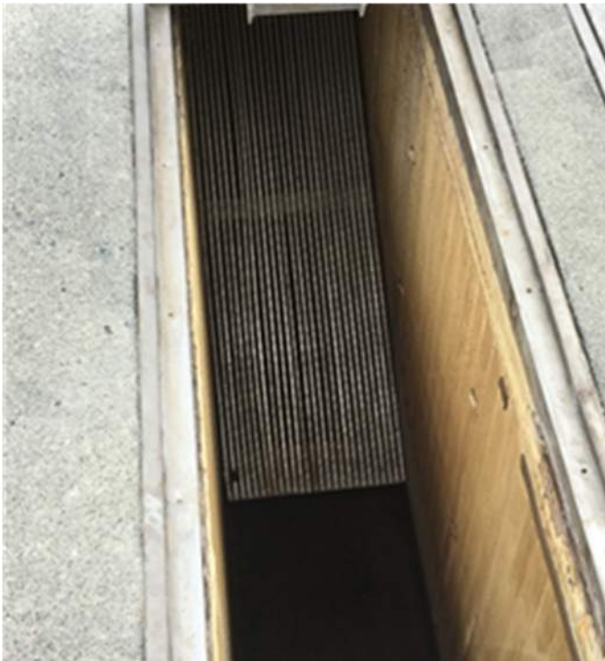
Photo 2: Bar Screen in Channel
