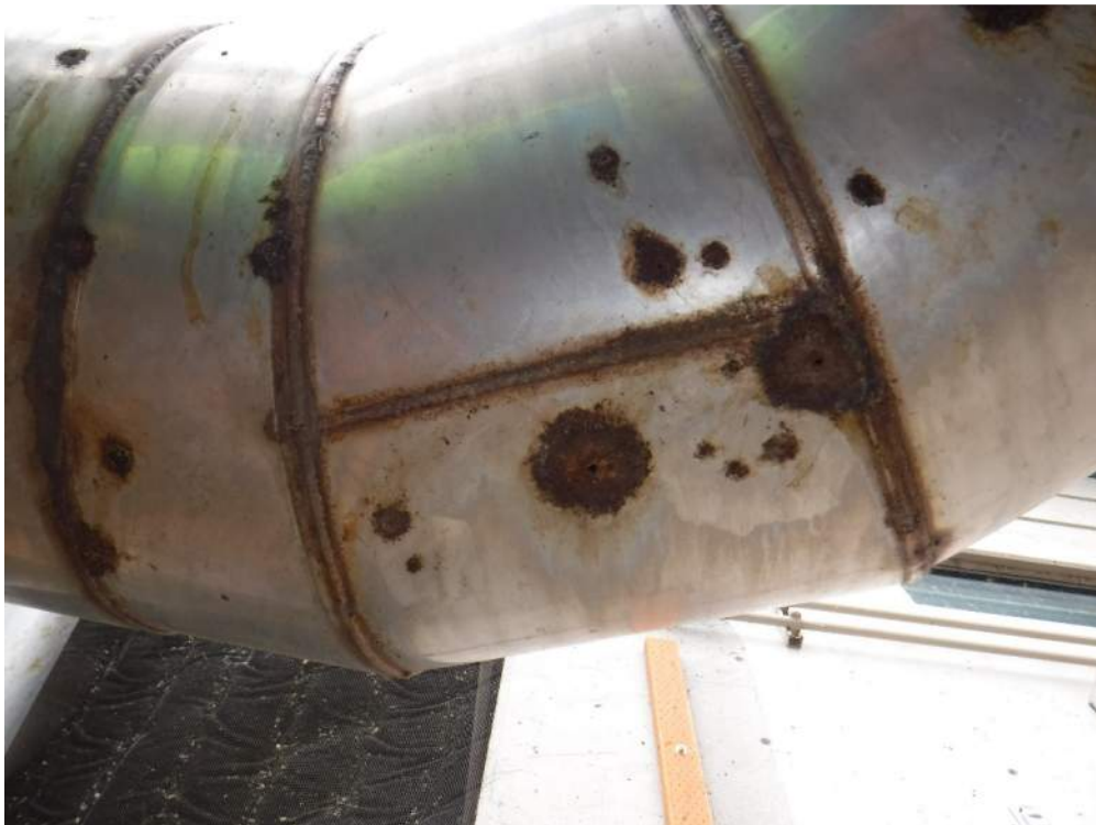
Photo 43. Typical penetrations in stainless steel odor control duct caused by internal corrosion.
