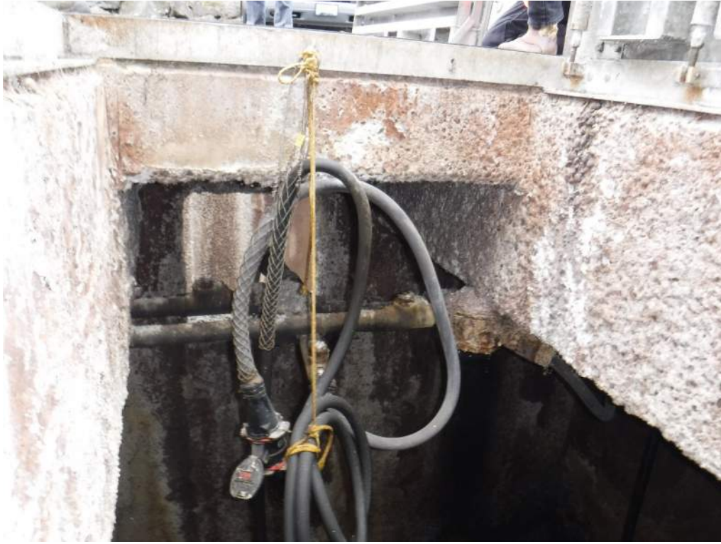
Photo 35. Deteriorated concrete and electrical components, influent wet well. Aluminum covers and stainless steel embeds are in good condition.
