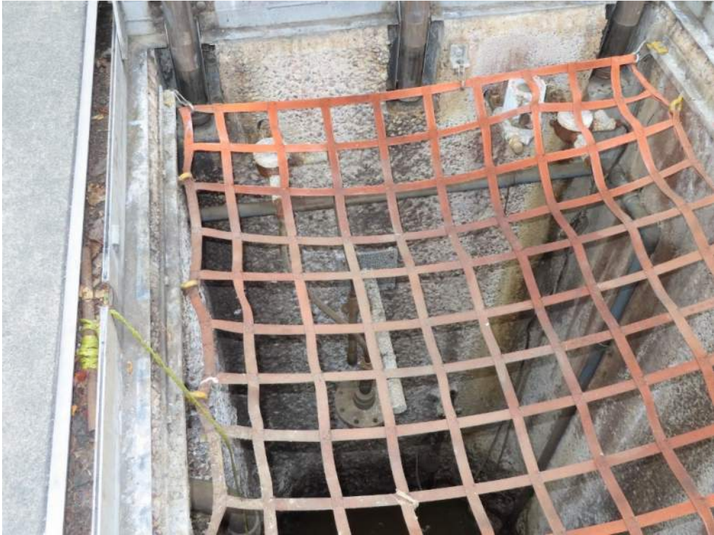
Photo 27. Gas transmitter experiences extreme corrosion
