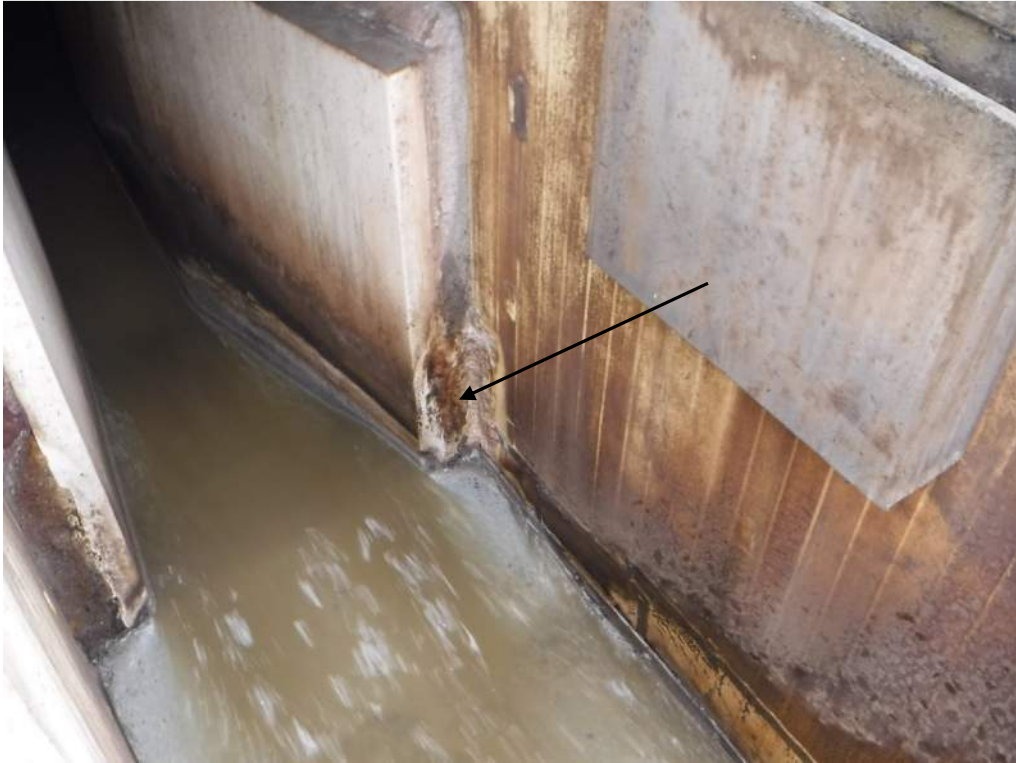
Photo 37. Concrete is corroding at base of Parschall Flume where embedded liner is ineffective (arrow).
