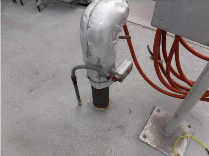
Photo 40. W3 line corroding wher it is not insulated. Not corrosion on conduit fittings (typical)
