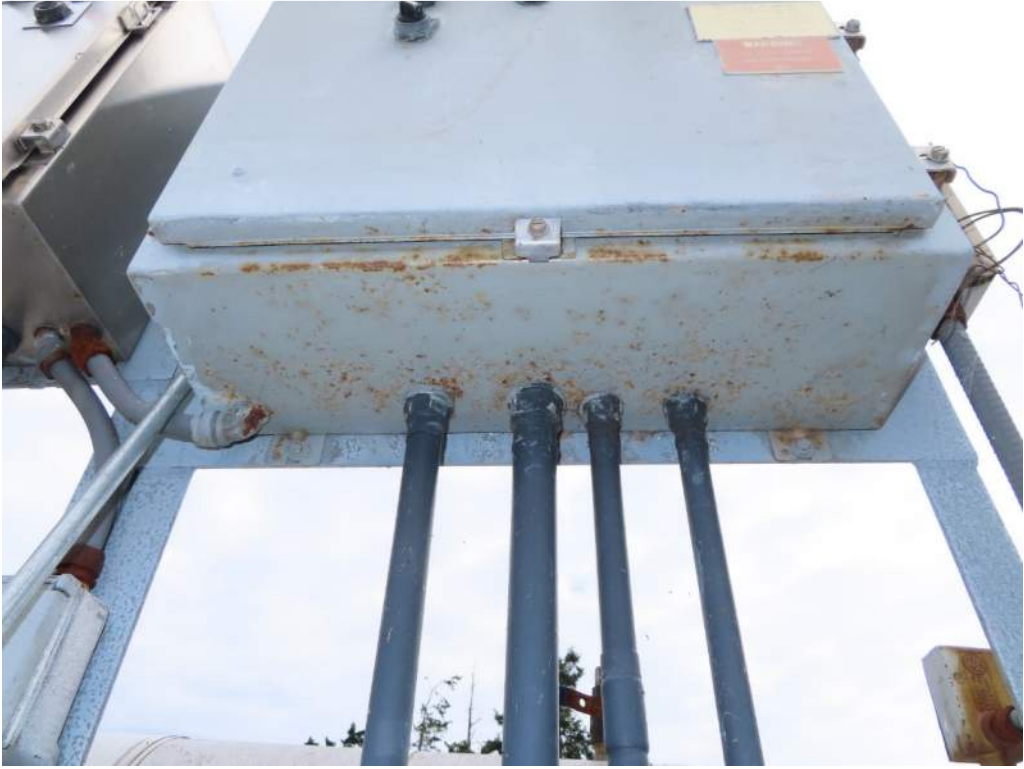
Photo 29. Corrosion of conduits and enclosures located outside
