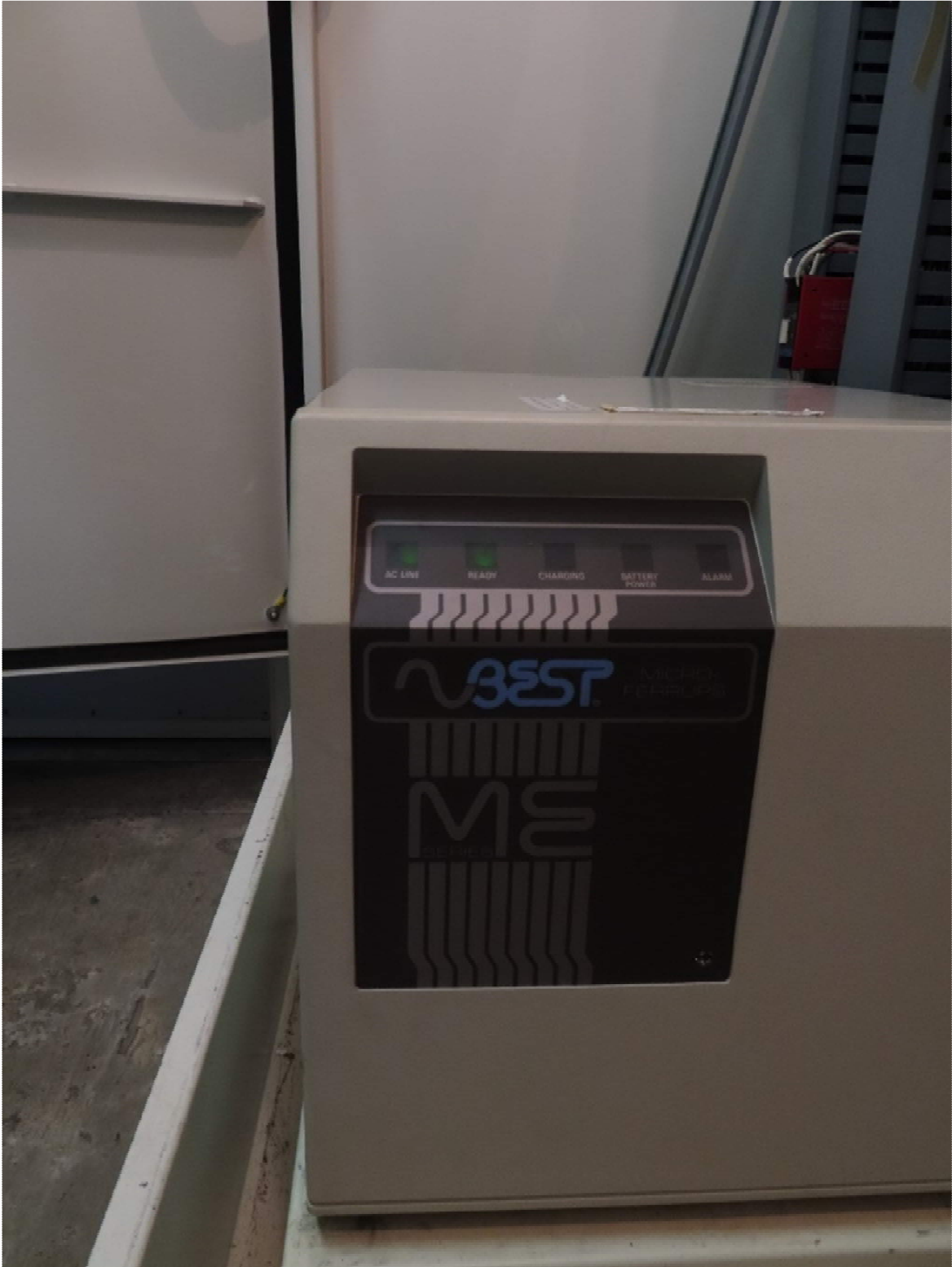
Photo 26. Conditions of UPS
