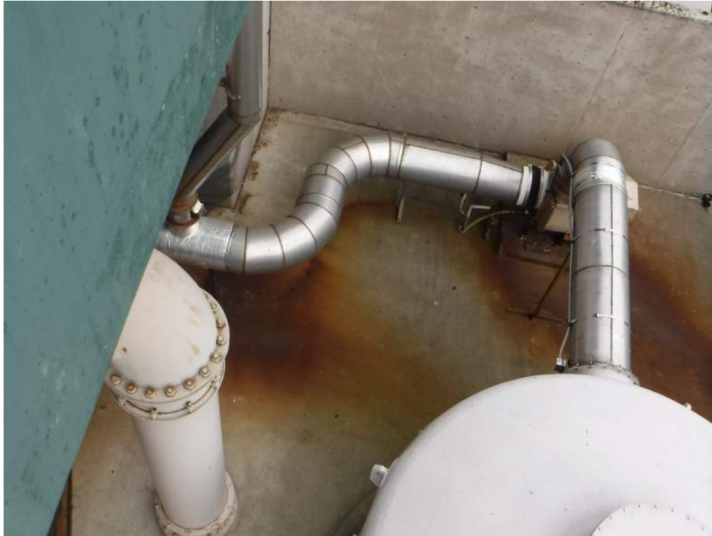
Photo 42. Rust staining on concrete floor under stainless steel odor control duct with penetrations caused by internal corrosion.
