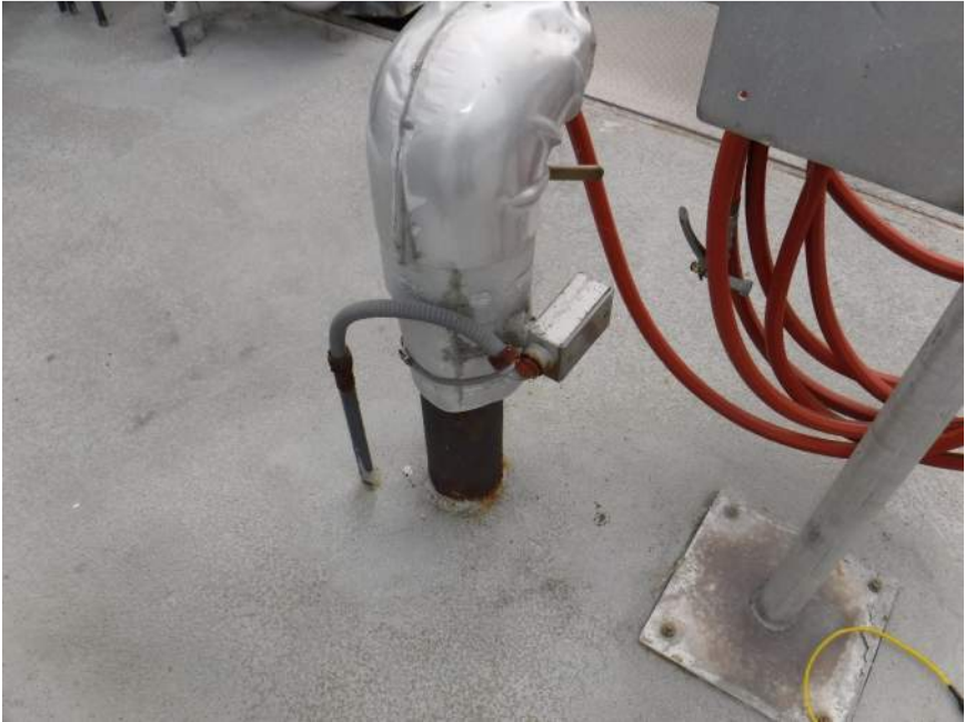
Photo 40. W3 line corroding wher it is not insulated. Not corrosion on conduit fittings (typical)
