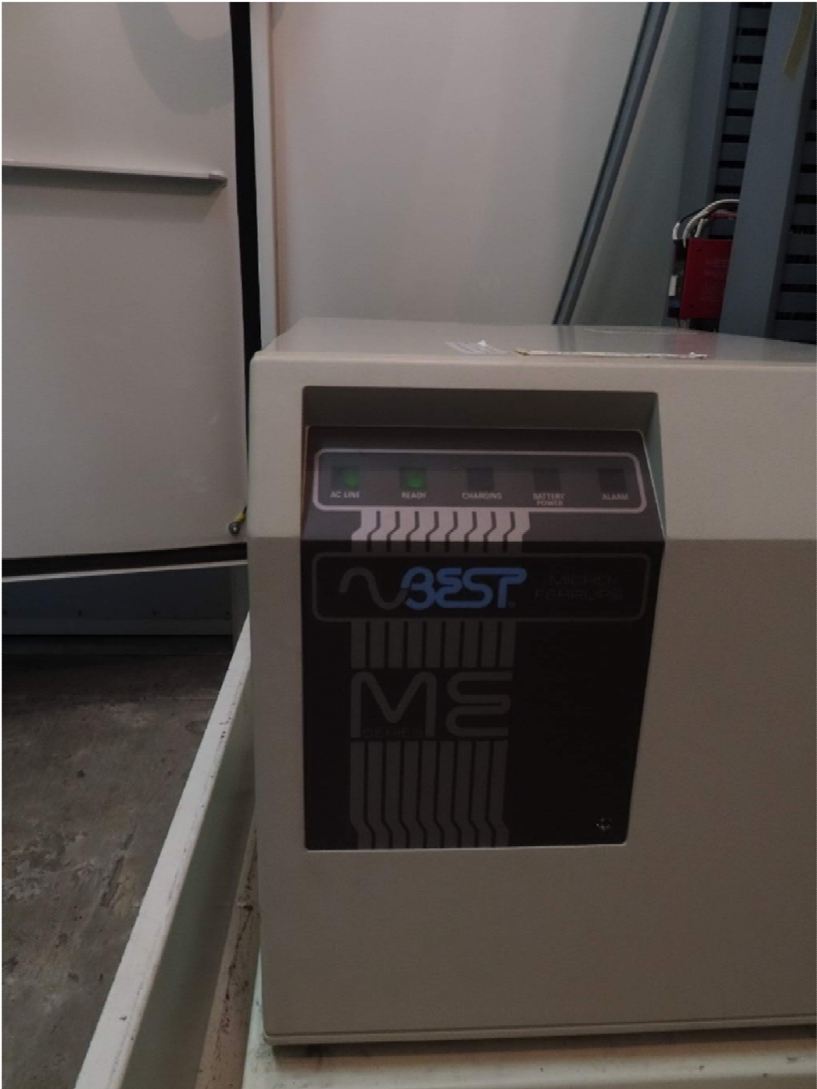
Photo 26. Conditions of UPS
