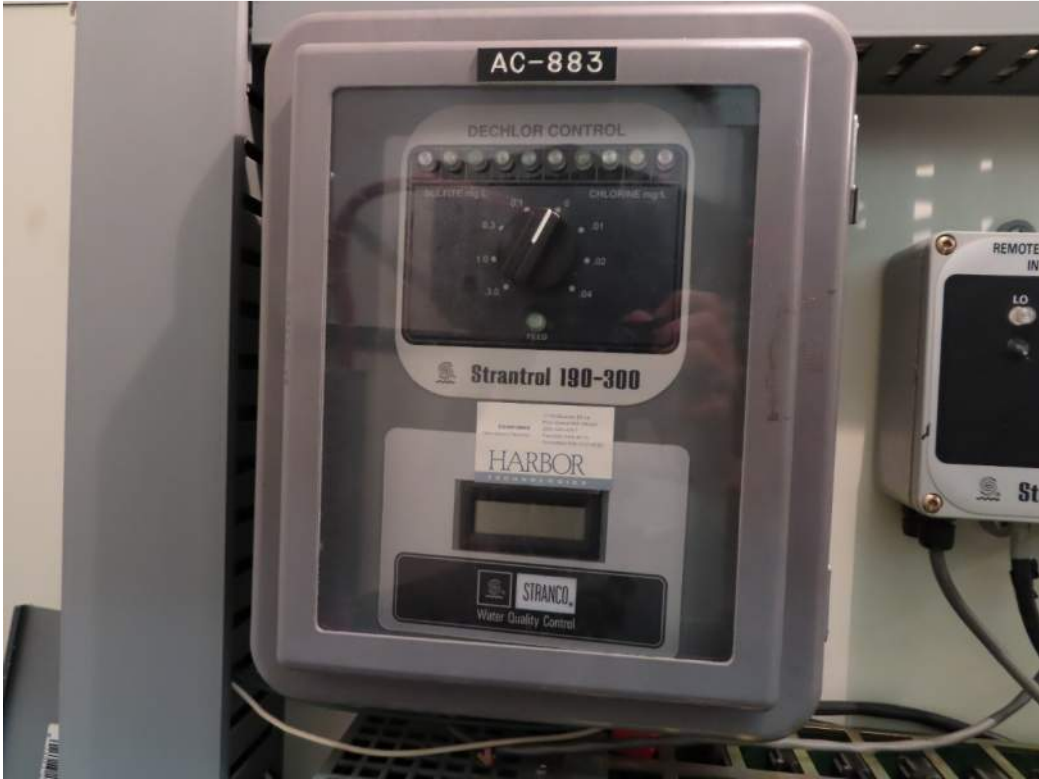
Photo 33. Deenergized Strantrol Dechlor controller
