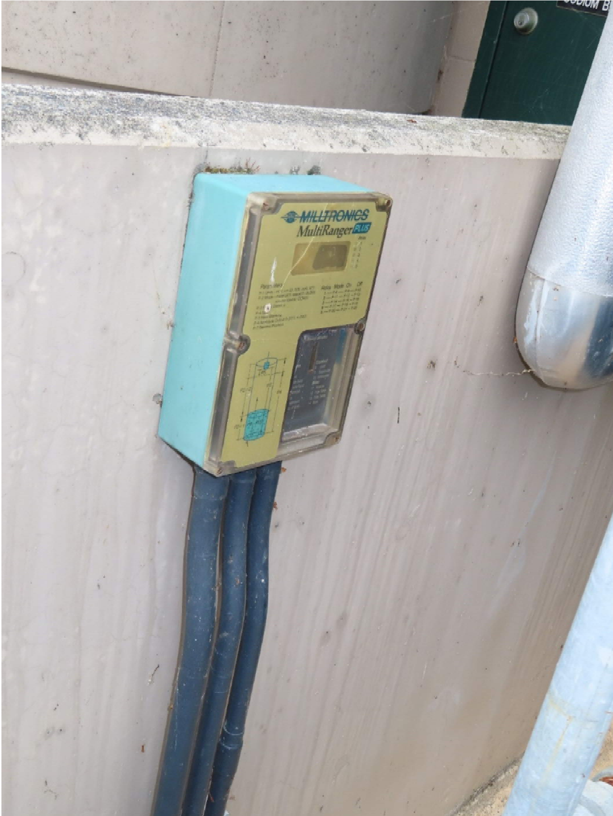
Photo 32. Abandoned the Milltronics transmitter
