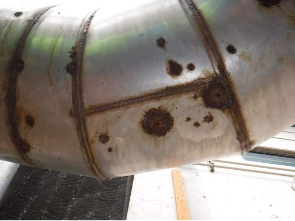
Photo 43. Typical penetrations in stainless steel odor control duct caused by internal corrosion.
