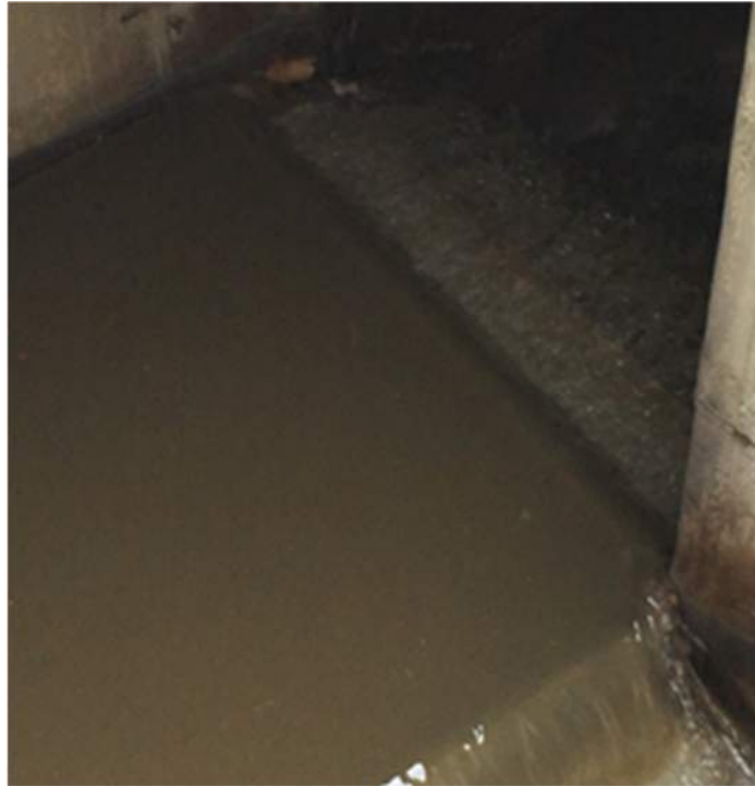
Photo 1: Oxidation Ditch Influent/RAS Splitter Box
