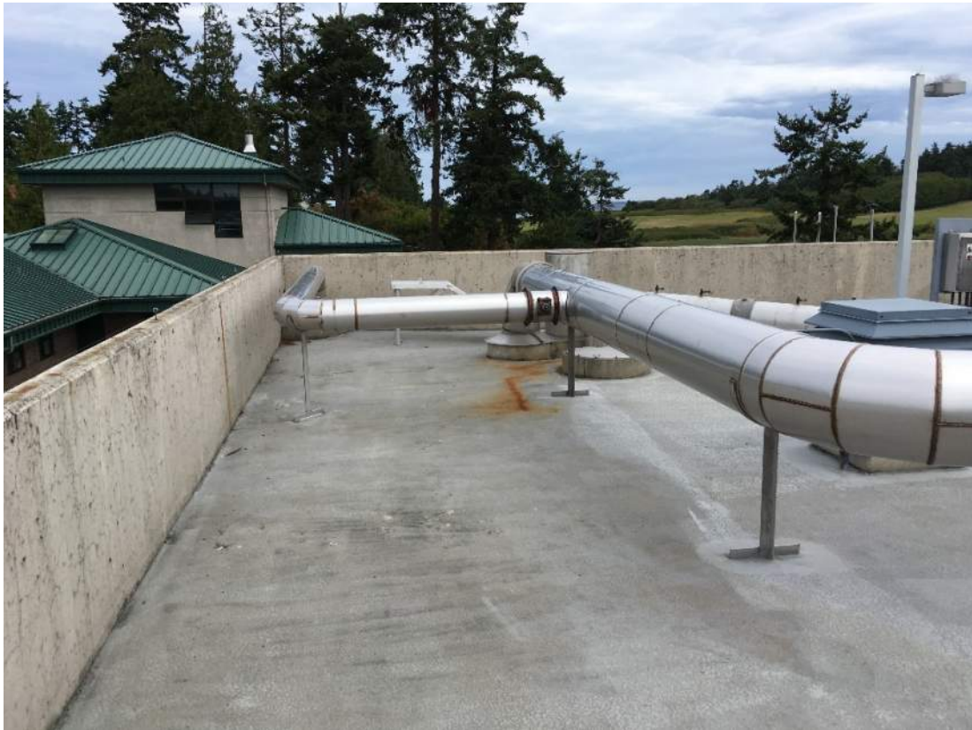
Photo 50: Route of Pump Around Over Parapet to Channel Upstream of Bar Screen and Odor Control Duct Down to Influent Pump Station.
