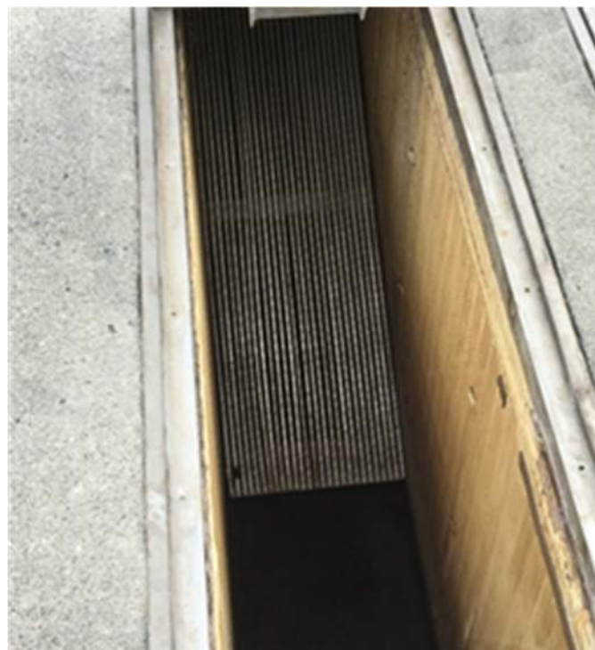
Photo 2: Bar Screen in Channel
