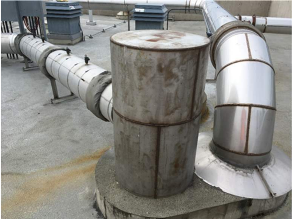
Photo 6: End of Screenings Compactor Tube and Odor Control Drawoff for Screenings and Grit Room
