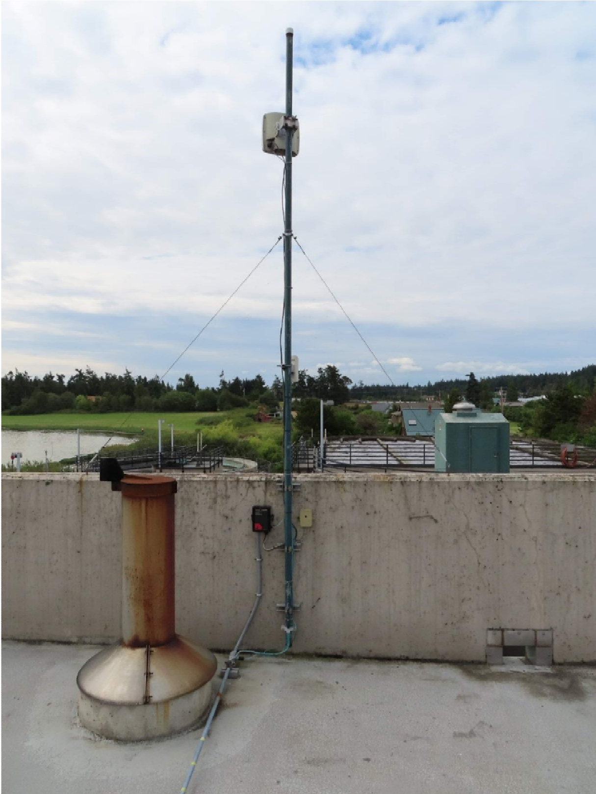
Photo 31. Abandoned network radio antenna
