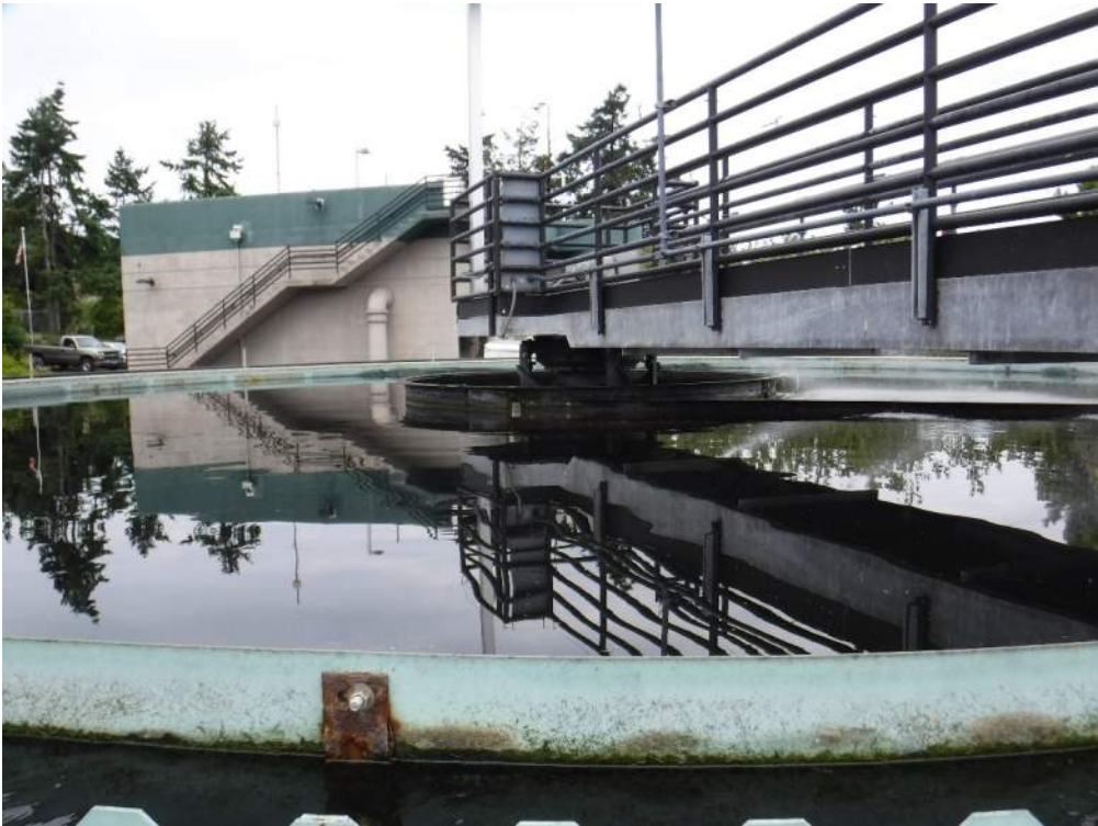
Photo 47. Corroding carbon steel baffle support bracket, north secondary clarifier.
