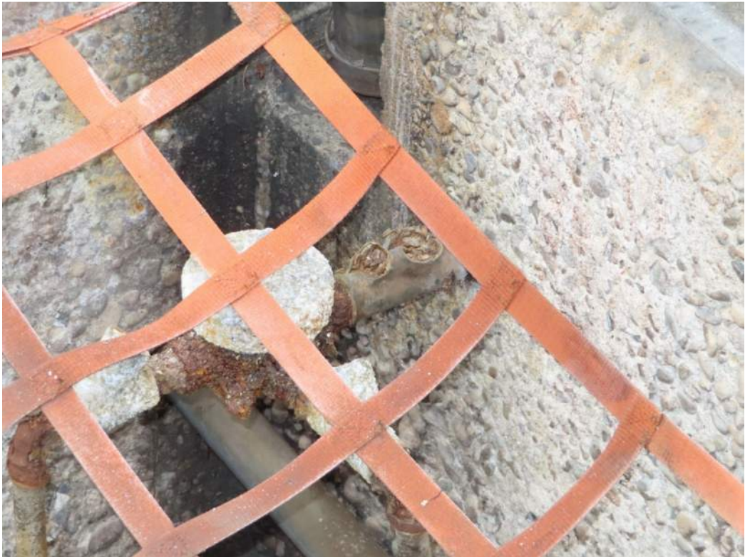
Photo 28. Gas transmitter experiences extreme corrosion
