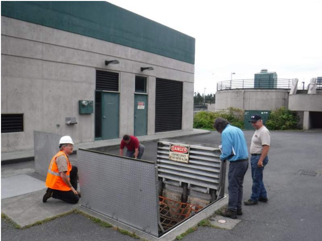
Photo 34. Influent Pump Station, Port Townsend wastewater treatment plant.
