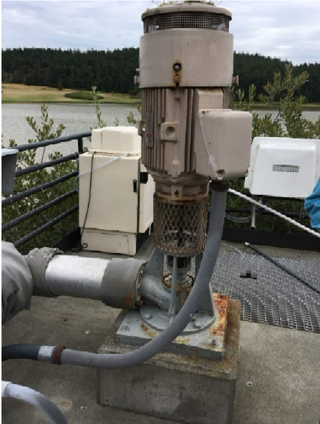
Photo 16: W3 pump and Effluent Sampler
