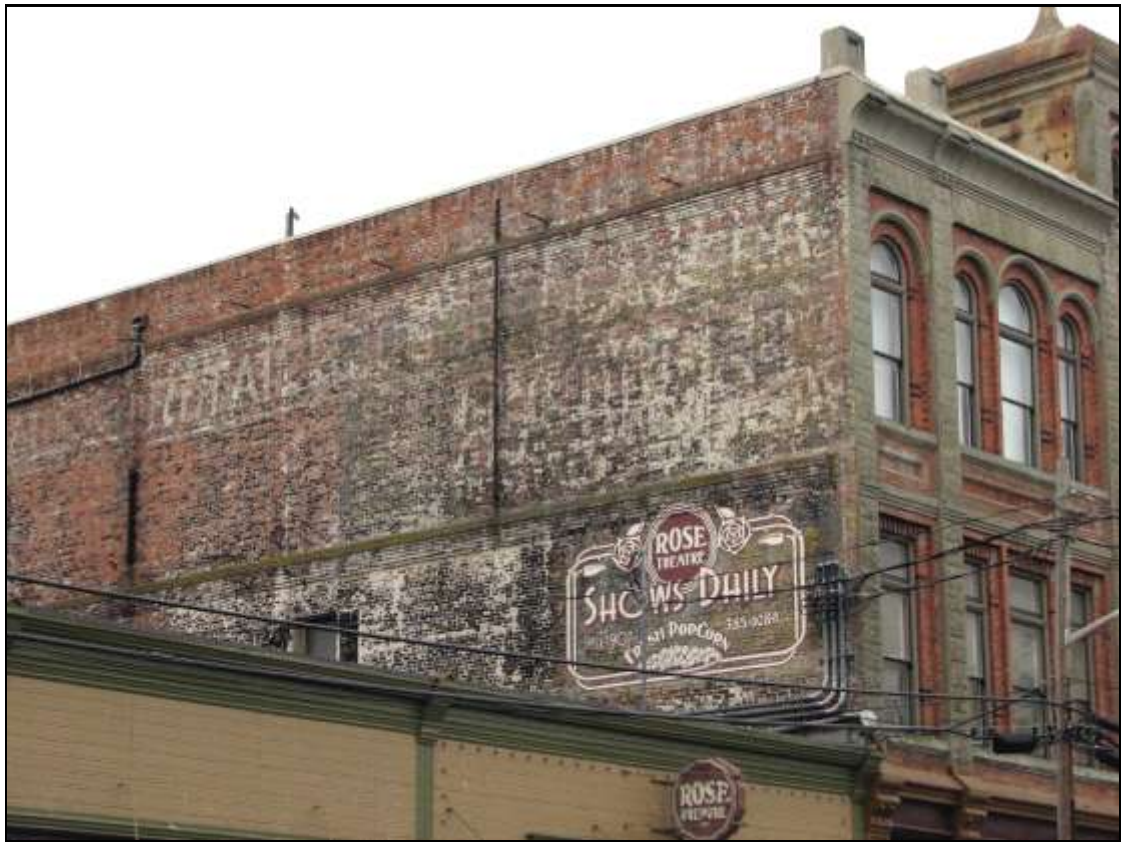
Miller Burkett Building's faded murals and a recently added mural for the Rose Theatre, November, 2010.
