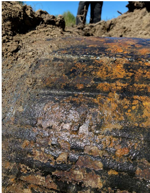
!928 Section at the Airport Illustrating Coating Loss – Photo Summer of 2020
