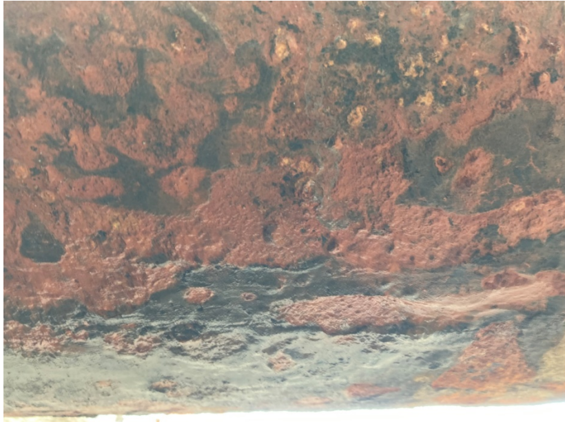
1928 Section of Pipeline at City CT Connection – 20" underside of pipe 10 feet from valve. Illustrates pitting in steel measure at approximately 0.09 inches.
