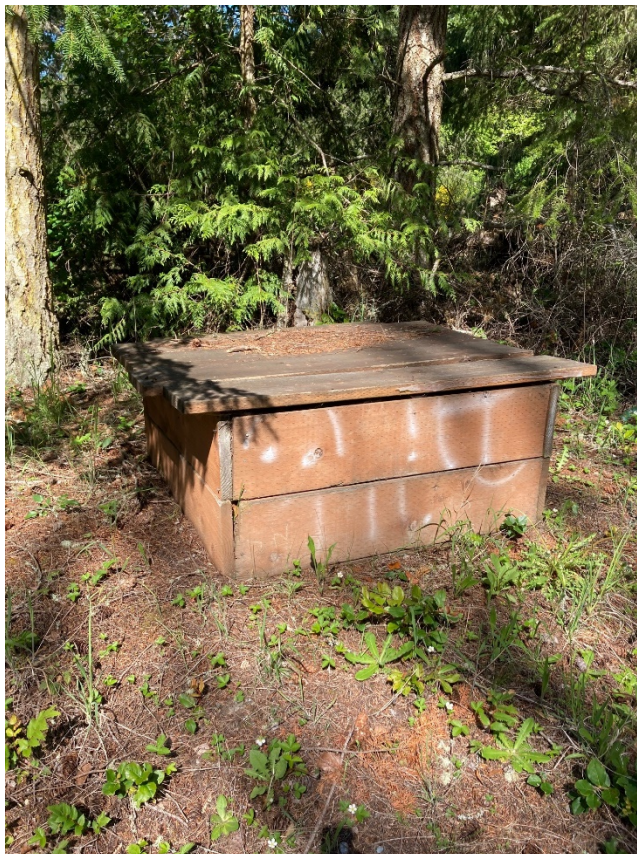
Air Valve Box
