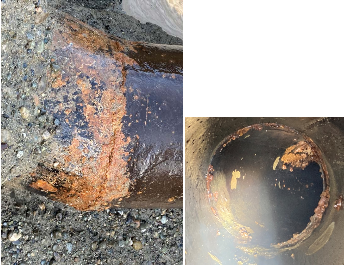
1928 Section of Pipeline at City CT Connection – 20" Mitered bend approx. 10 feet from valve. Illustrates weld condition and coatings failure on exterior of pipe (LT) and interior weld corrosion and small coating failures on inside of pipe (RT).
