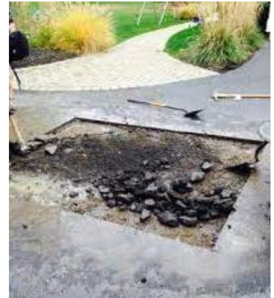
Hot asphalt patching and repair result in long term better outcomes rather than cold mix patching
