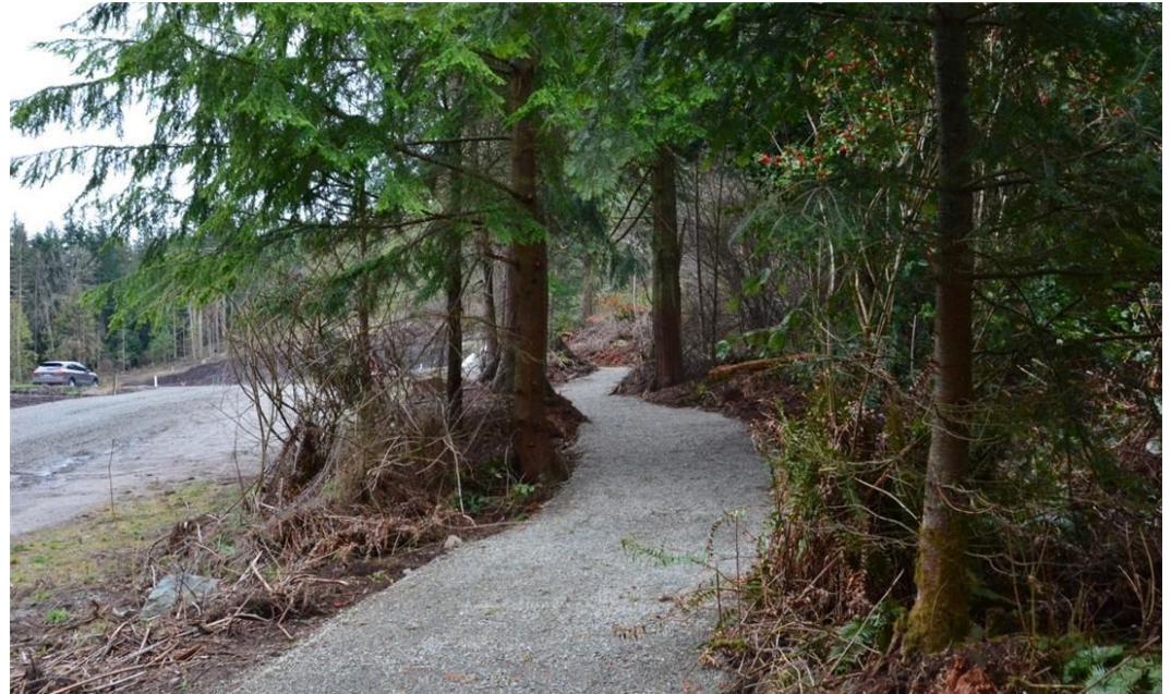
Example of trail and a road being built as part of the Trail Crest Development
