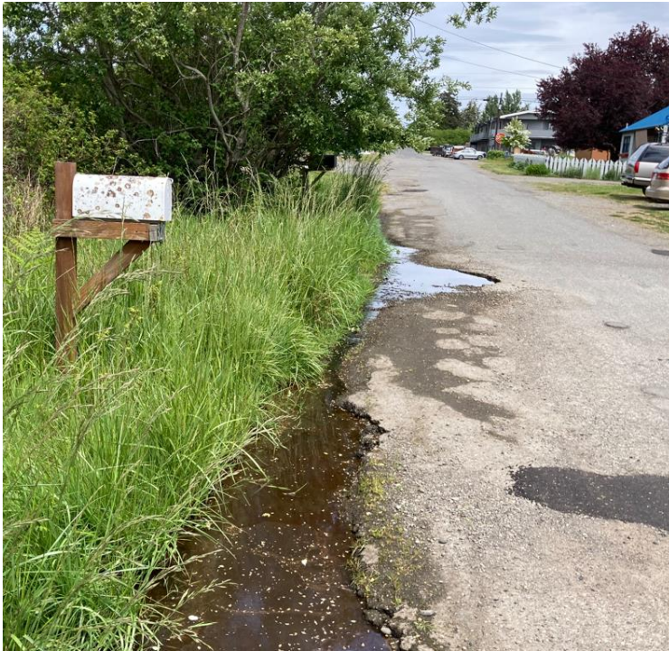
Asphalt deterioration due to drainage on Hancock Street
