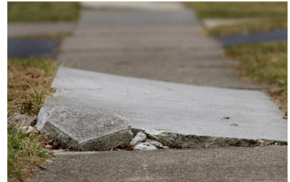
Sidewalk Trip Hazards
