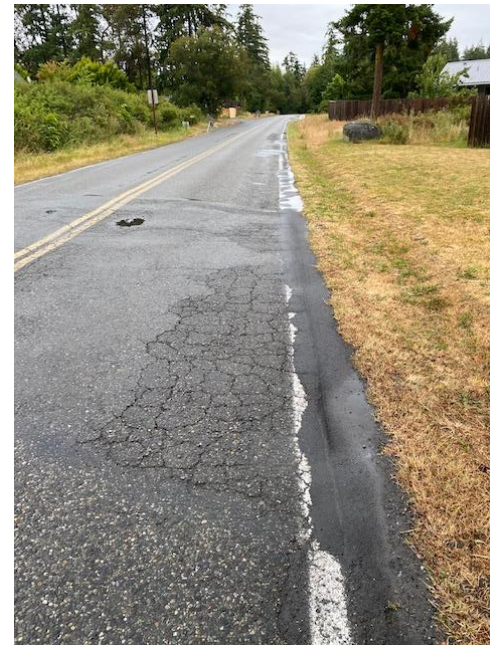
Street edge failure due to lack of stormwater drainage. Streets often fail from the outside in.
