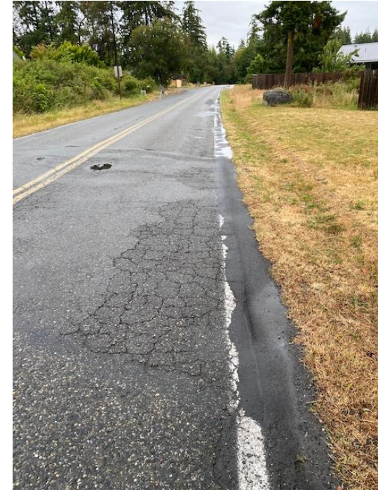
Shoulder Failure Alligator cracking: Discovery Road
