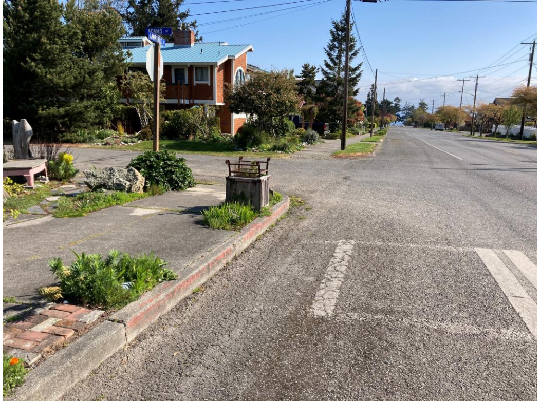
Lawrence Street & Adams Street - Missing Wheelchair Ramp
