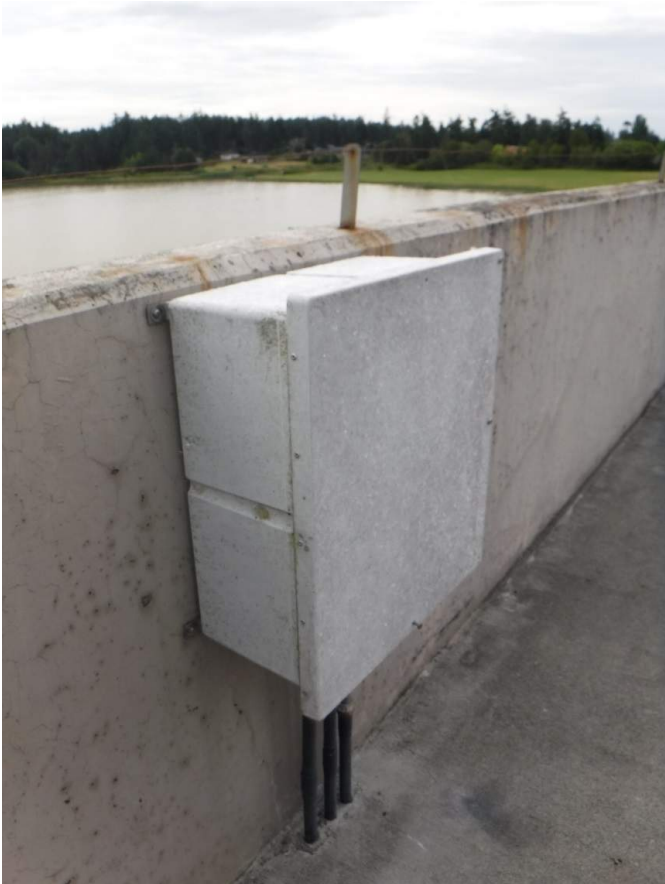
Photo 41. Fiberglass box housing instrument panel, subject to UV deterioration (east side of headworks).
