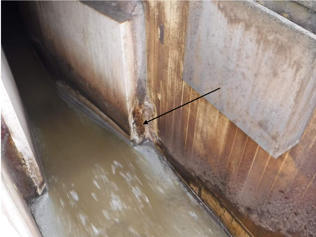
Photo 37. Concrete is corroding at base of Parschall Flume where embedded liner is ineffective (arrow).
