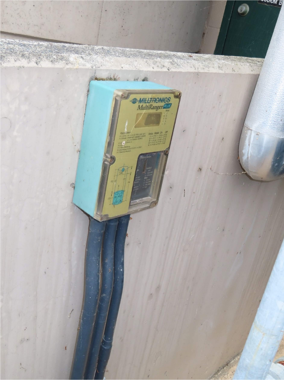
Photo 32. Abandoned the Milltronics transmitter
