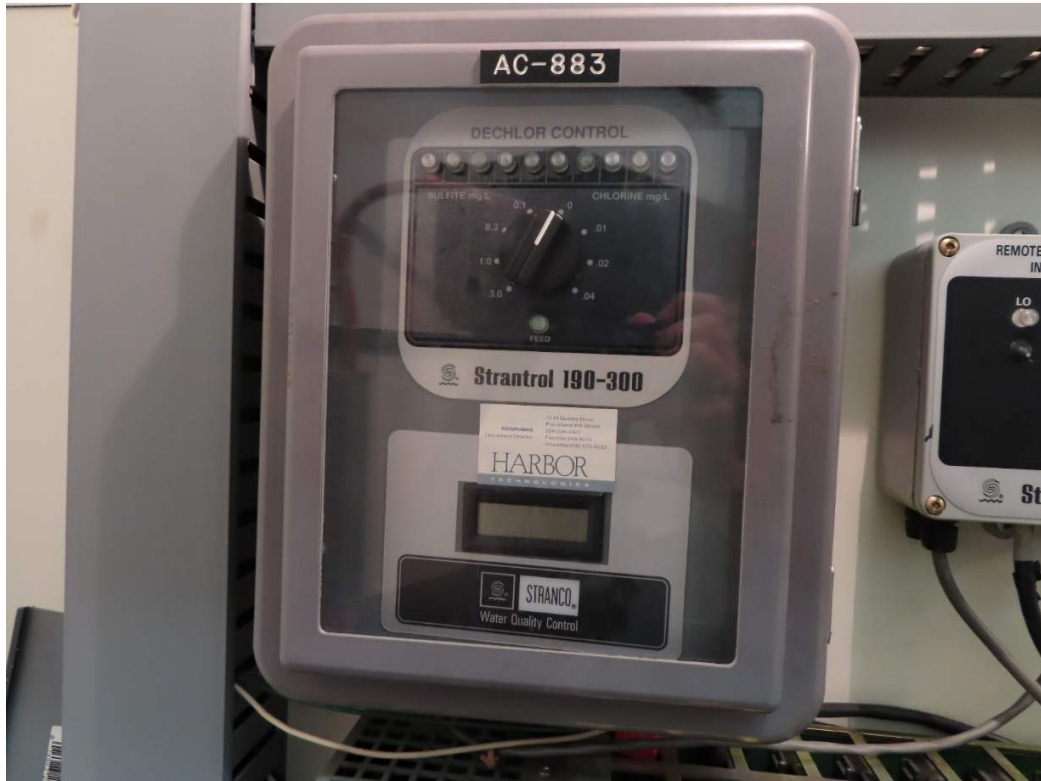
Photo 33. Deenergized Strantrol Dechlor controller
