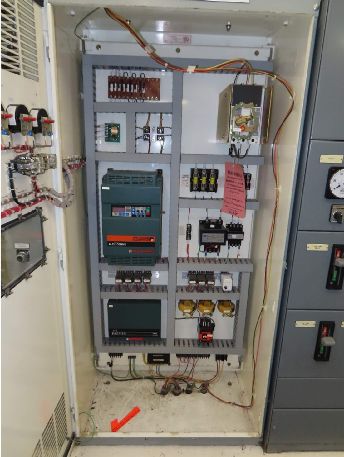
Photo 25. Conditions of VFD
