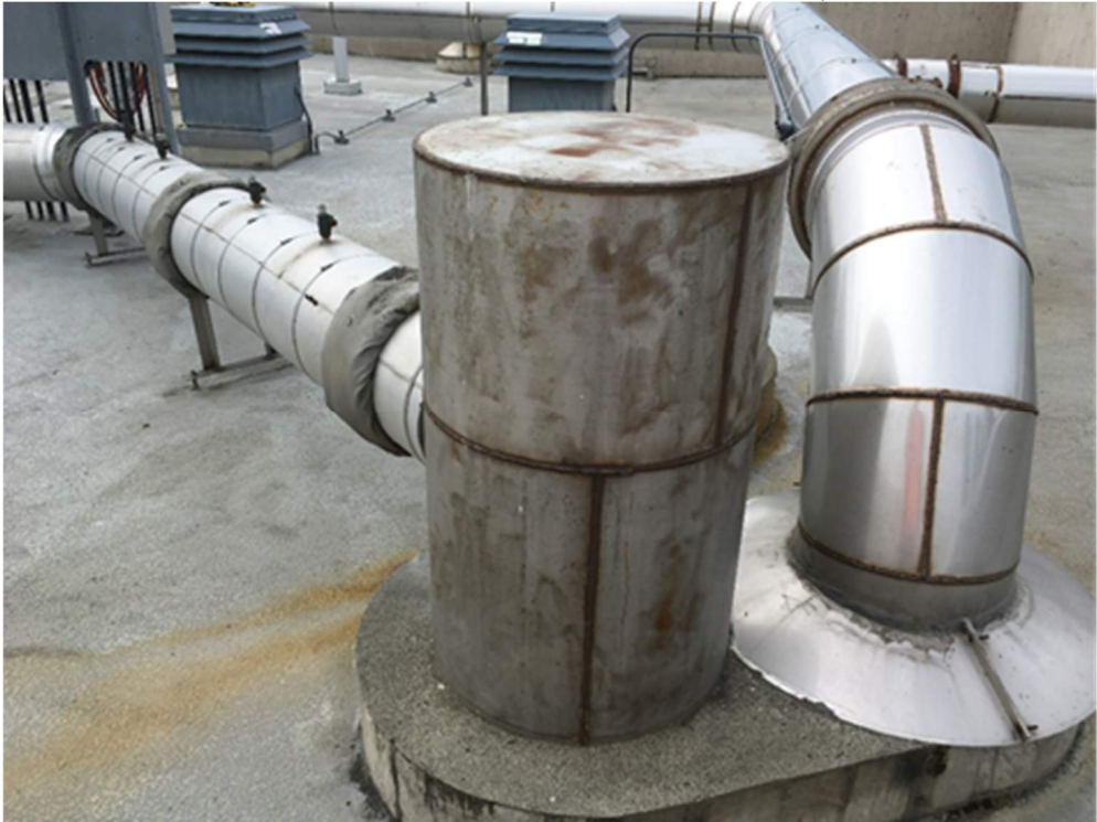
Photo 6: End of Screenings Compactor Tube and Odor Control Drawoff for Screenings and Grit Room
