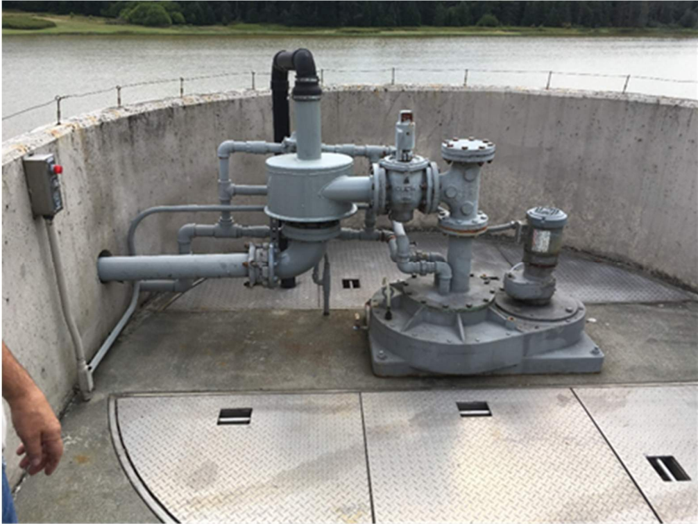
Photo 5: Pista Grit Drive Mechanism and Rebuilt Vortex Separator
