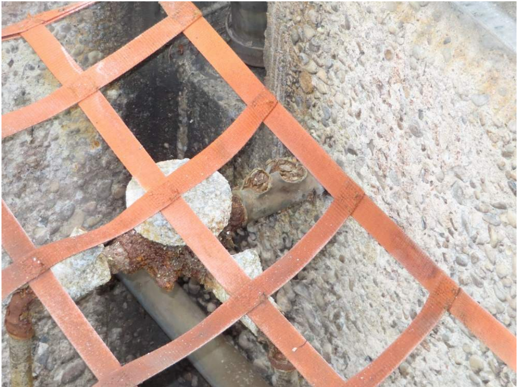
Photo 28. Gas transmitter experiences extreme corrosion
