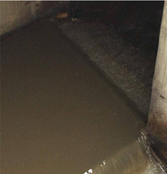
Photo 1: Oxidation Ditch Influent/RAS Splitter Box
