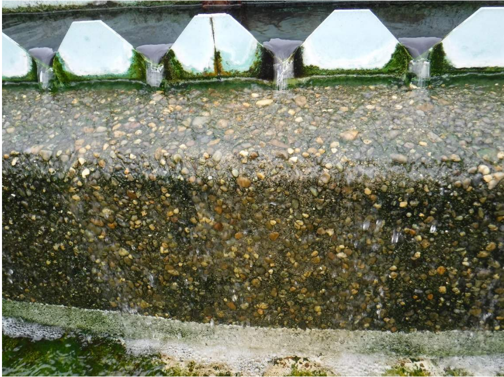
Photo 46. Exposed aggregate in launder, north secondary clarifier.
