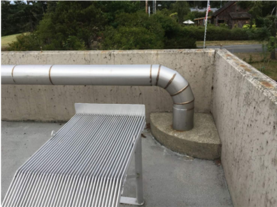
Photo 4: Manual Bar Rack
