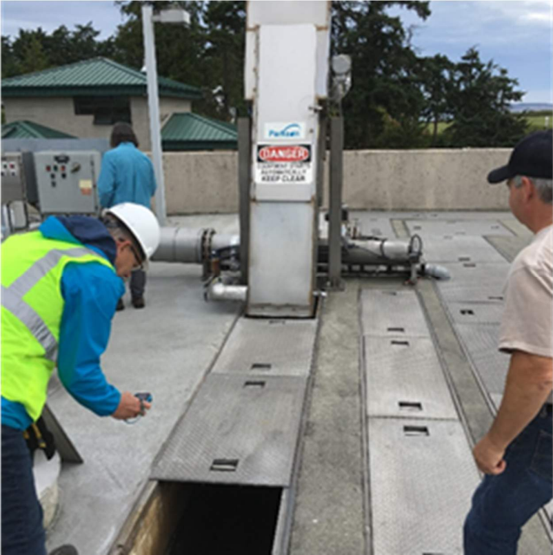
Photo 3: Bar Screen Enclosure and Compactor
