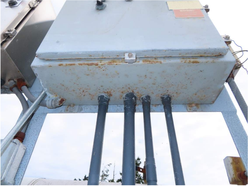
Photo 29. Corrosion of conduits and enclosures located outside
