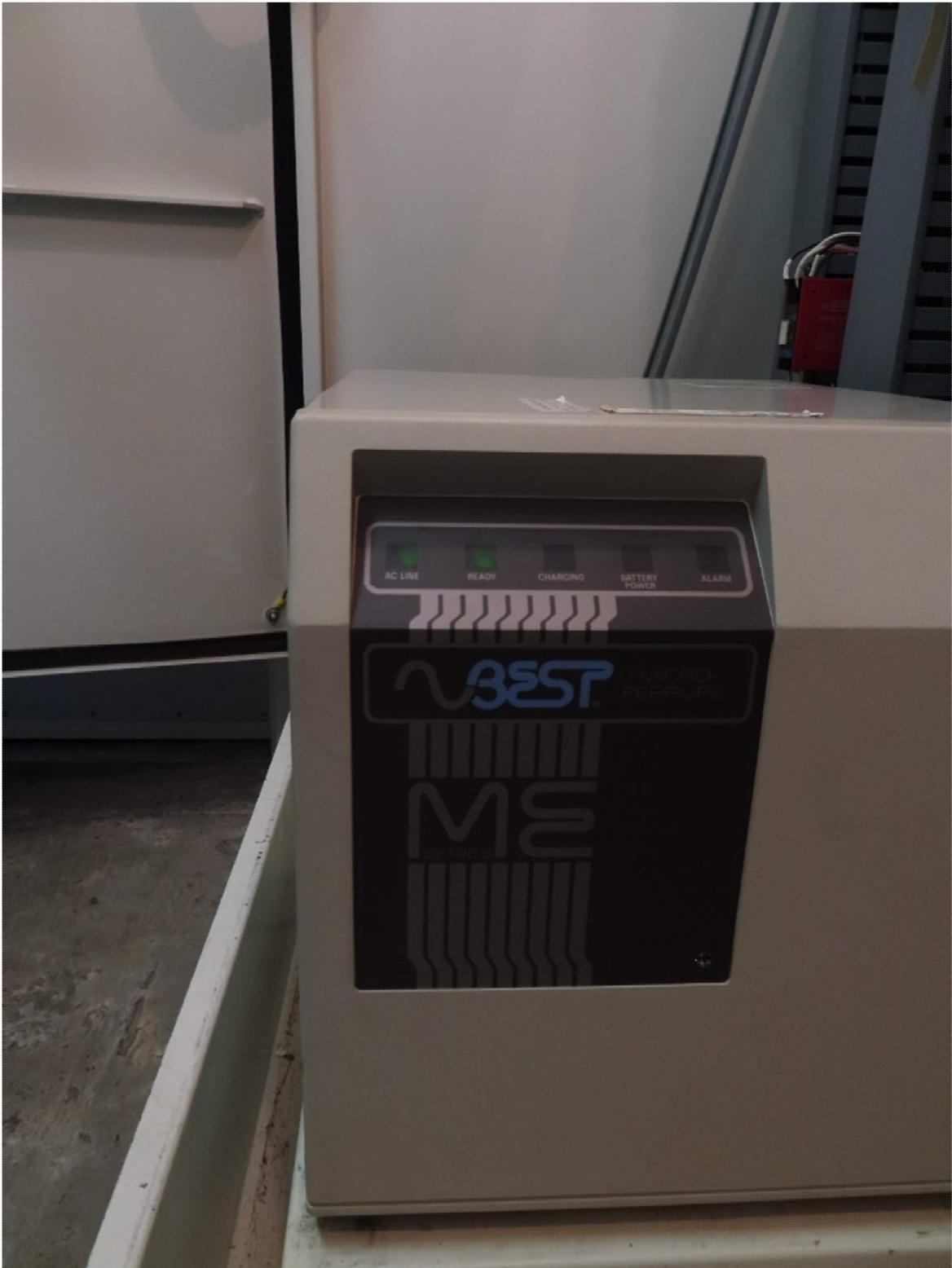
Photo 26. Conditions of UPS
