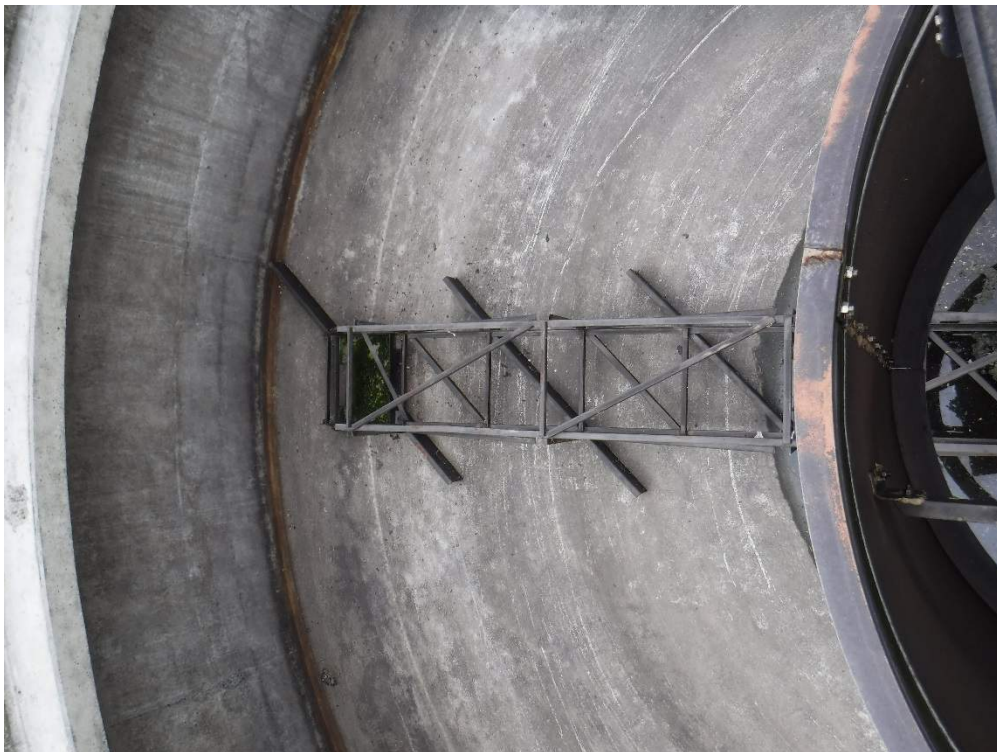
Photo 45. Clarifier mechanism rake arm and well. Note coating deterioration on top of well angle (red primer is showing). Some corrosion is occurring on rake arms where coating has failed.
