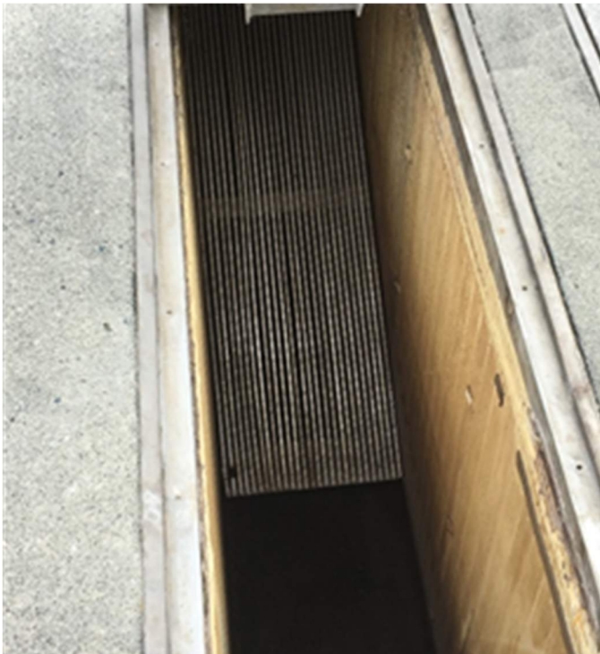
Photo 2: Bar Screen in Channel
