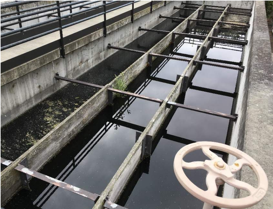
Photo 15: Chlorine Contact Basin
