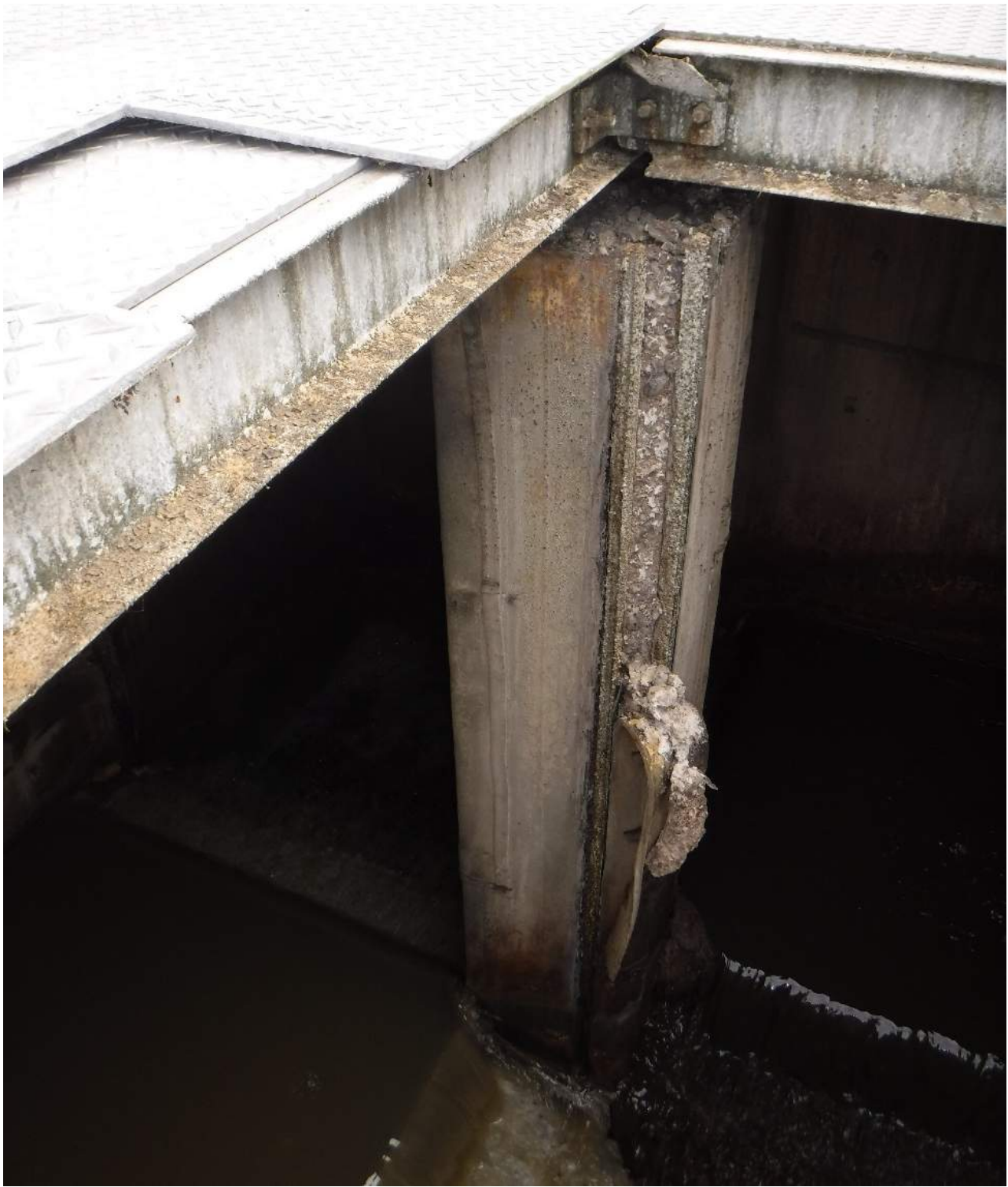
Photo 39. Failure of embedded liner on corners of concrete support column, RAS return basin.
