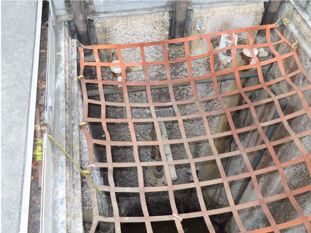
Photo 27. Gas transmitter experiences extreme corrosion
