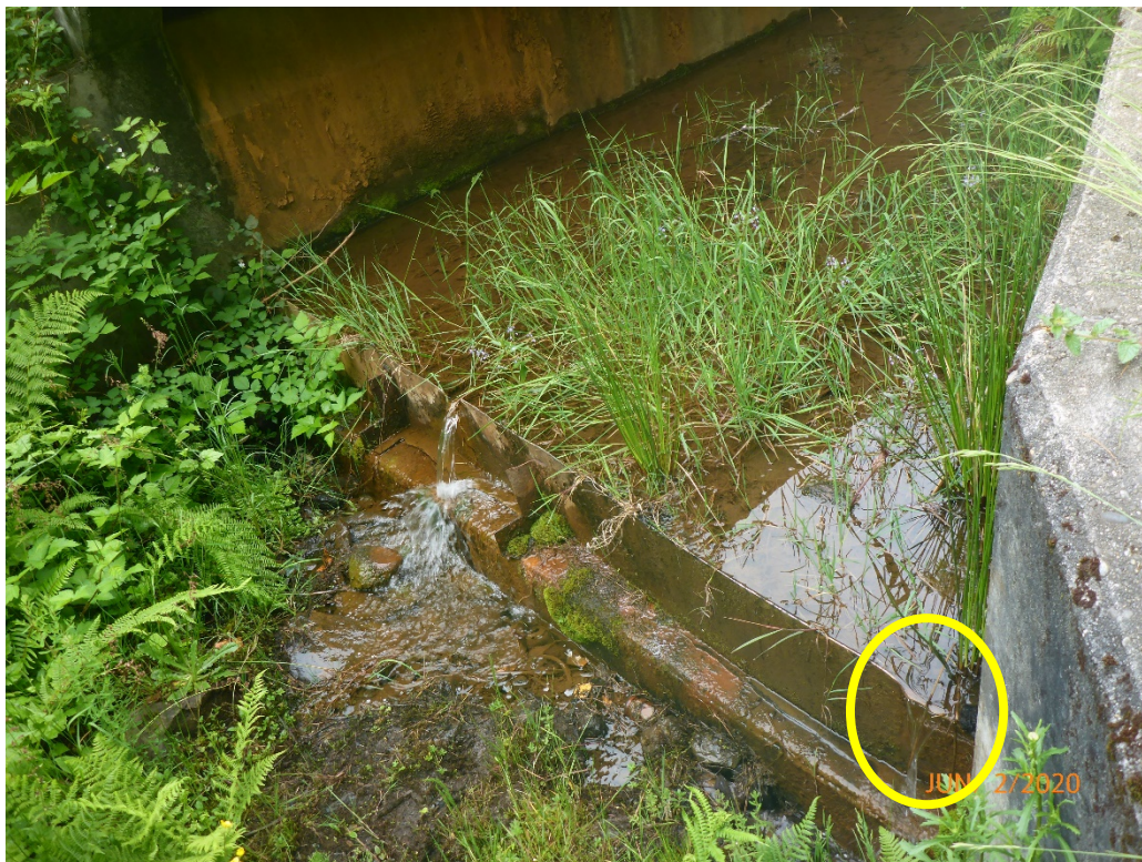
Photo 10: V-notch weir at seepage measurement point number 1. Damage section highlighted.
