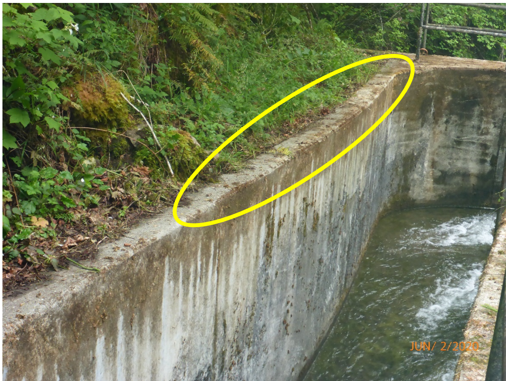
Photo 8: View of spillway at entrance channel. Concave area highlighted.
