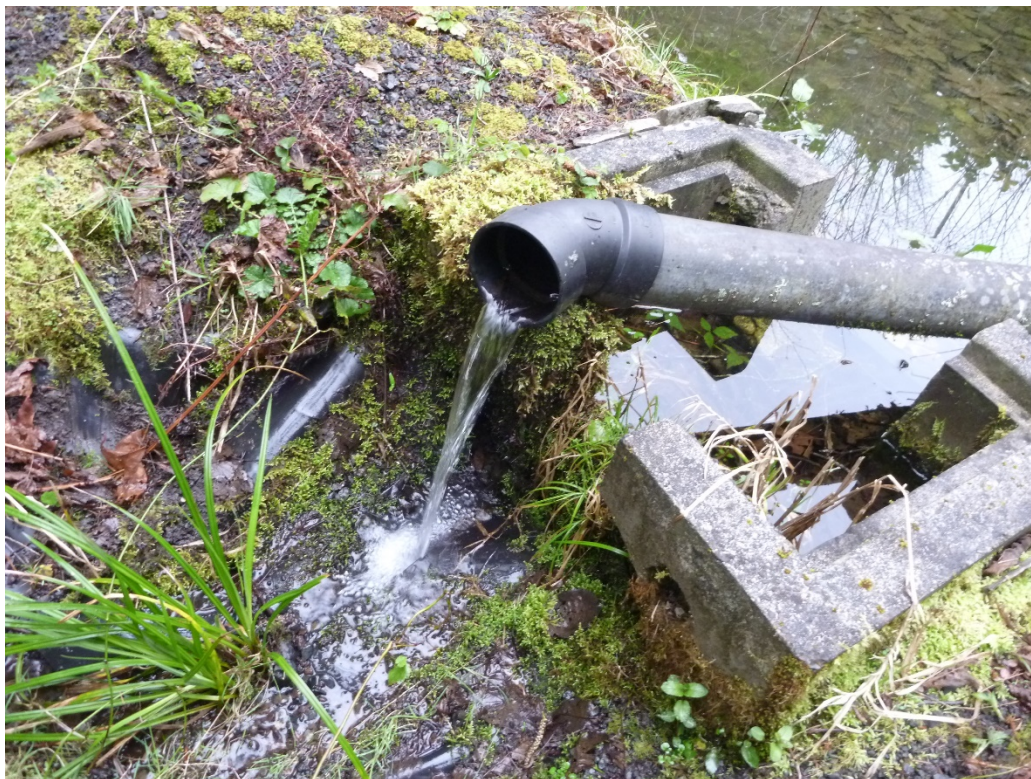
Photo 2: Weir and drain pipe at downstream toe area of North Dam during 2015 DSO inspection.
