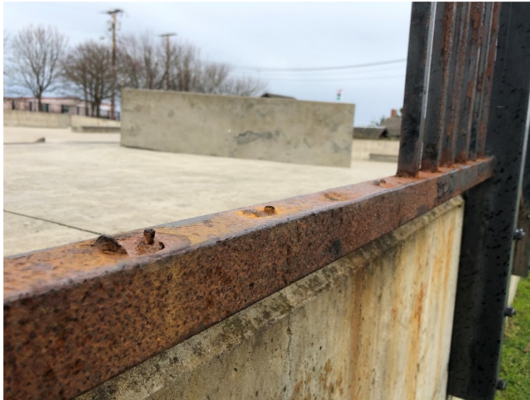
Photo of Typical Corrosion
