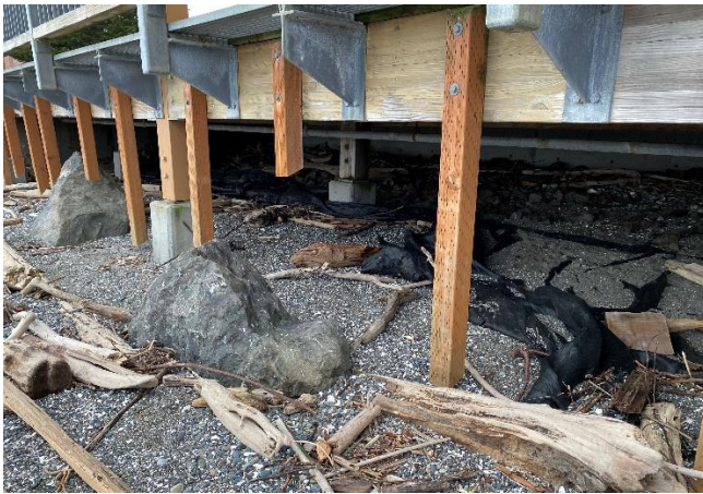
H. Damage and debris under deck after 1/13/21 storm.
