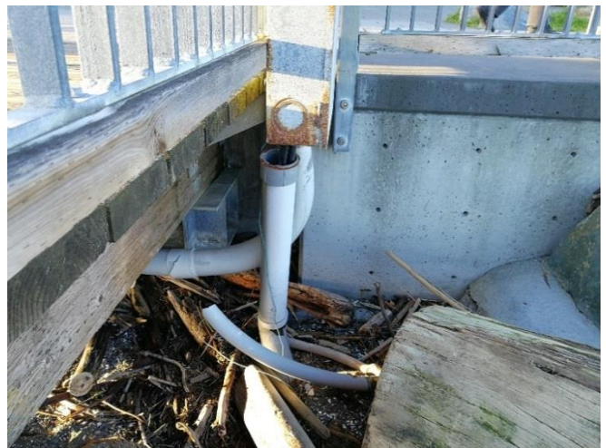
F. Damaged electrical box and HDPE wire conduit
