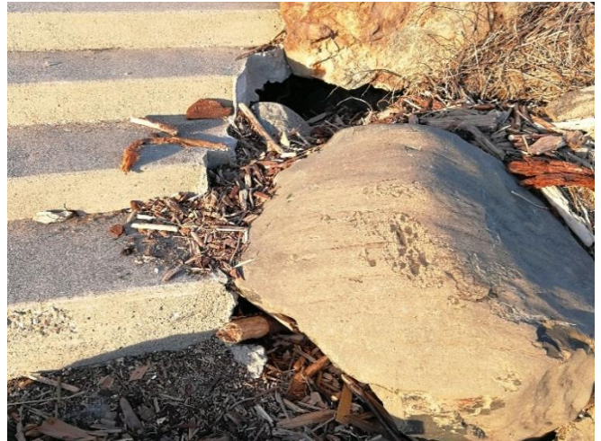
D. Displaced landscaping boulder and voids
