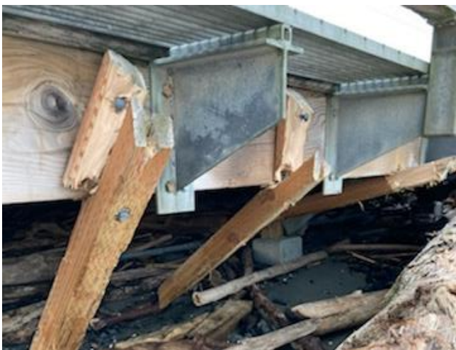
J. Damage and debris under deck after 1/7/22 storm.
