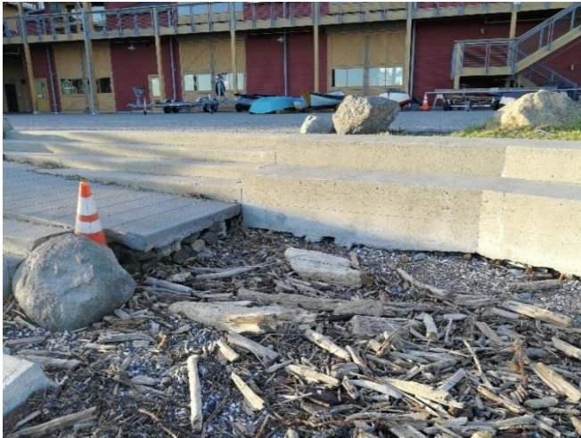
C. Scour and exposed base of concrete stairs
