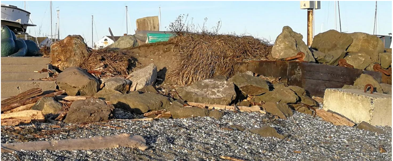
G. Under-protected and eroded bank northeast of concrete stairway from 12/20/18 storm event at the project area.
