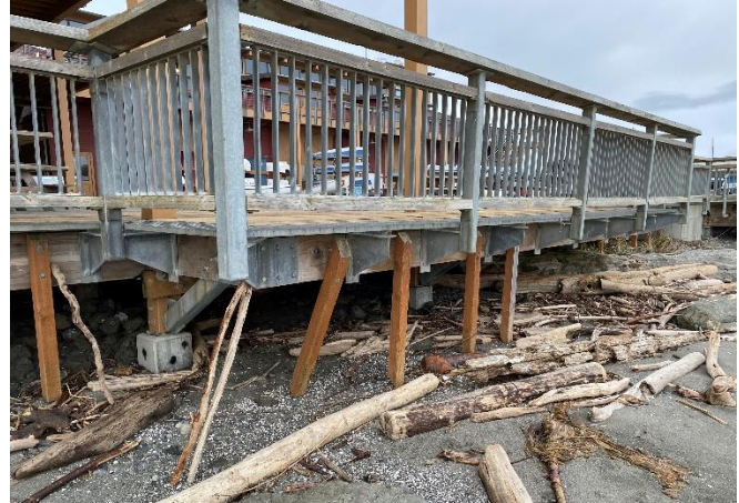
I. Damage and debris under deck after 1/13/21 storm.
