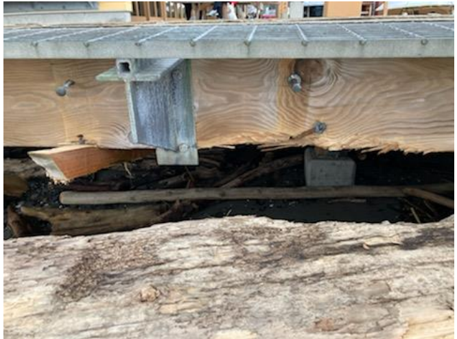
K. Damage and debris under deck after 1/7/22 storm.
