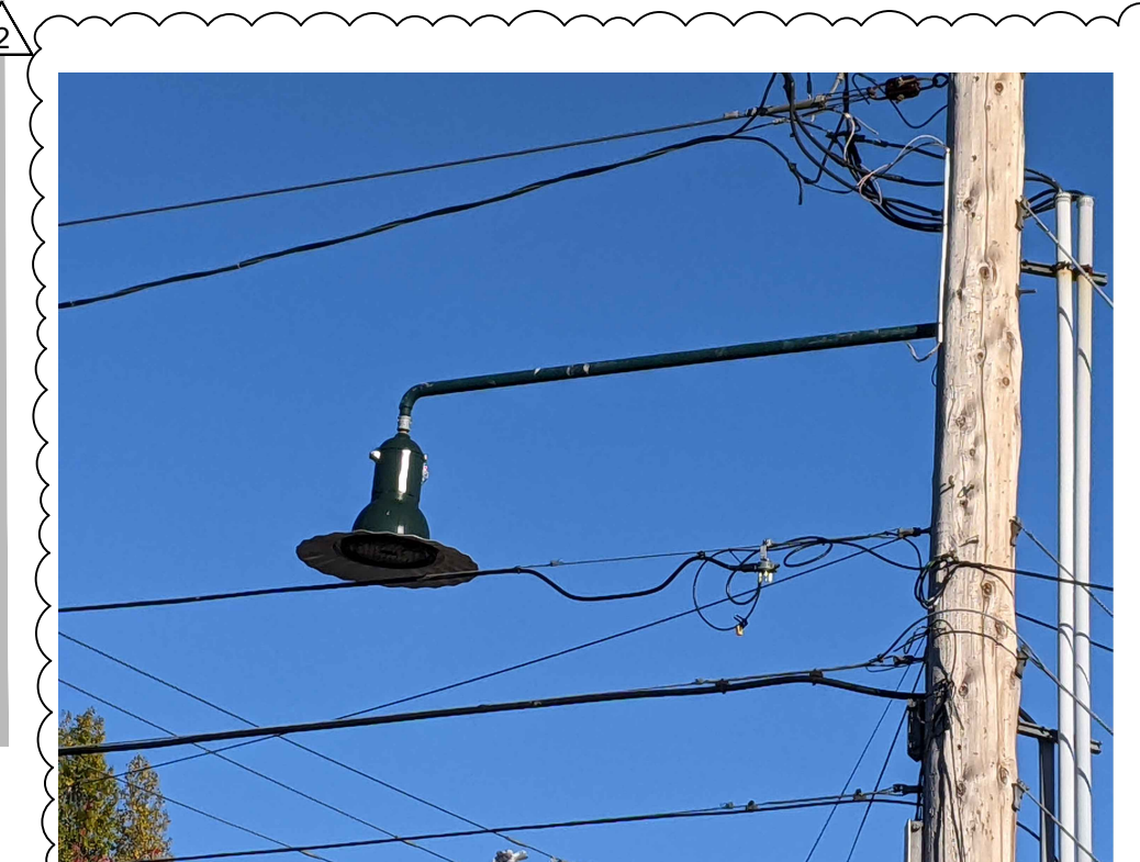
EXAMPLE OF STREET LIGHT FOR LOCATIONS ON SAN JUAN AVENUE OR DISCOVERY (SAME AS EXISTING FIXTURE AT SAN JUAN - DISCOVERY INTERSECTION)
