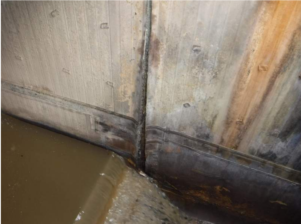
Photo 38. Embedded liner pulling from concrete at temporary gate groove, RAS return basin.
