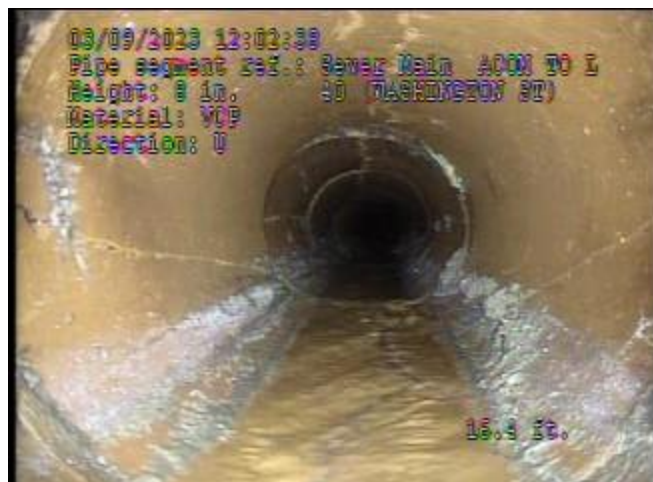
Longitudinal cracks and deformation in Washington Street sewer portend collapse.
