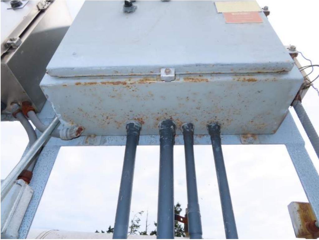
Photo 29. Corrosion of conduits and enclosures located outside
