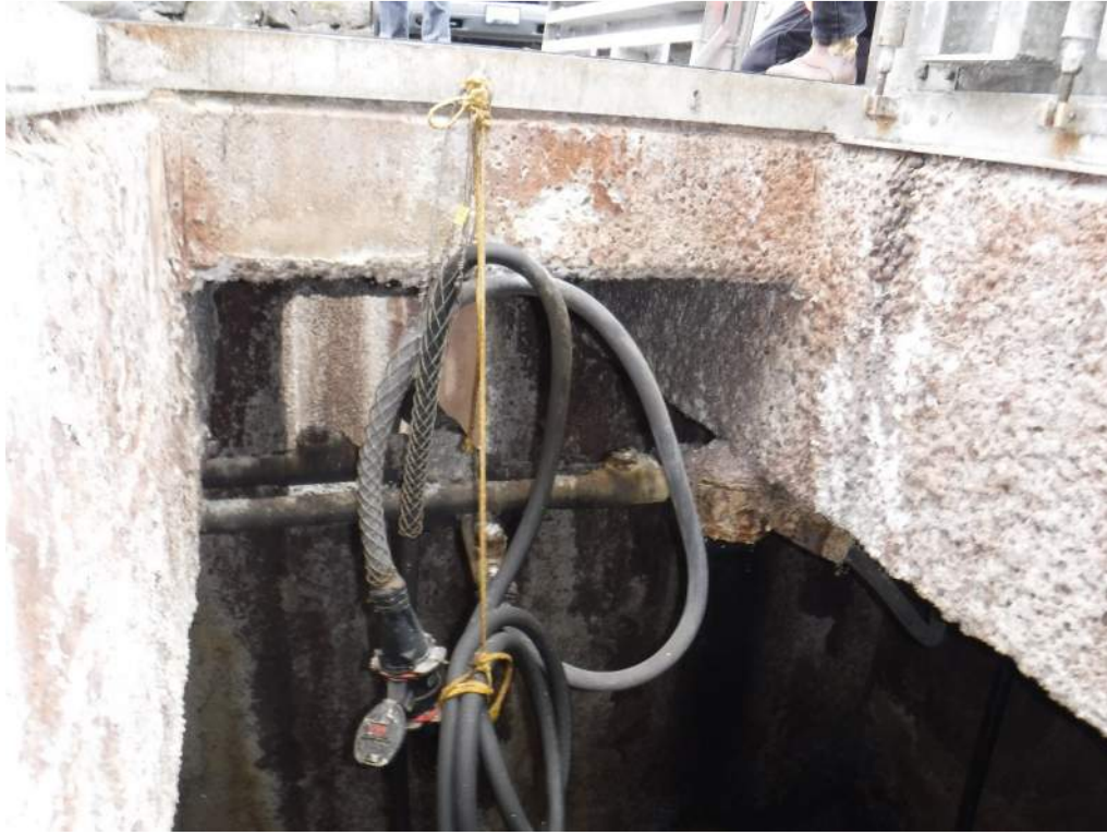
Photo 35. Deteriorated concrete and electrical components, influent wet well. Aluminum covers and stainless steel embeds are in good condition.
