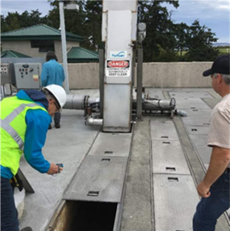
Photo 3: Bar Screen Enclosure and Compactor
