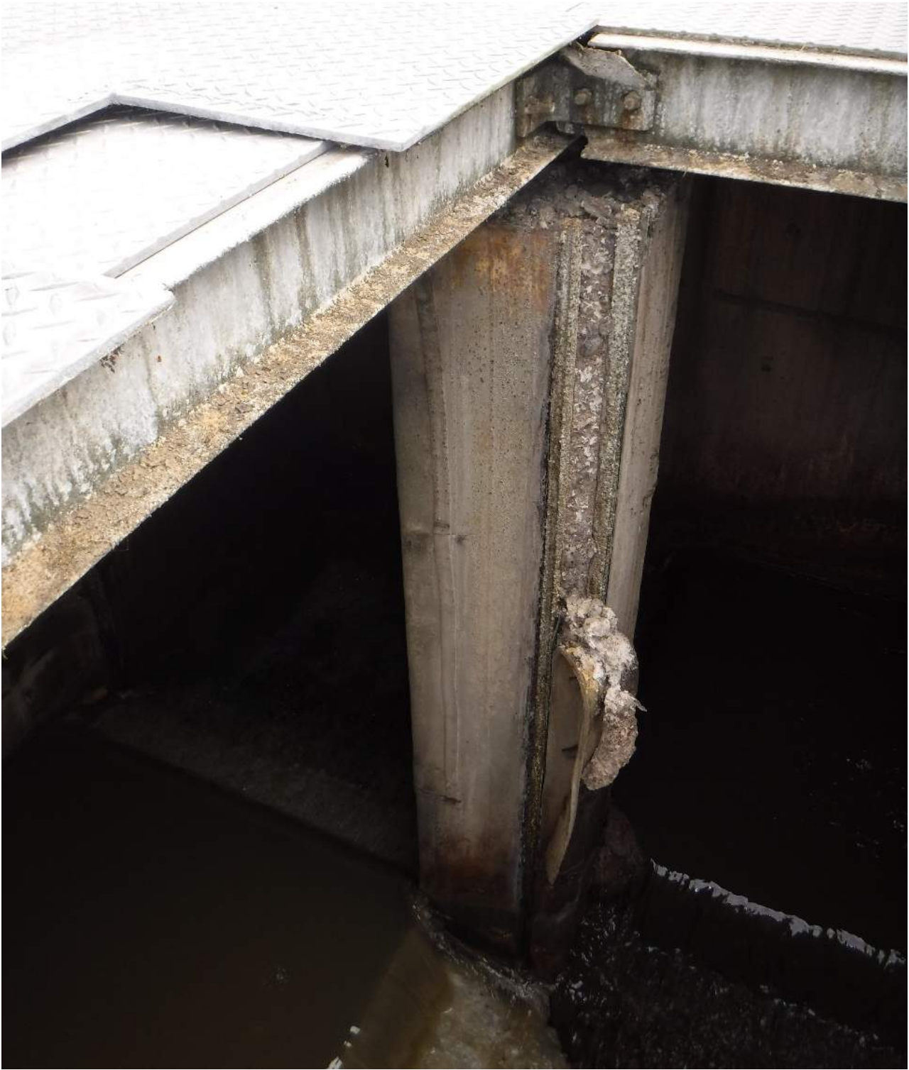
Photo 39. Failure of embedded liner on corners of concrete support column, RAS return basin.
