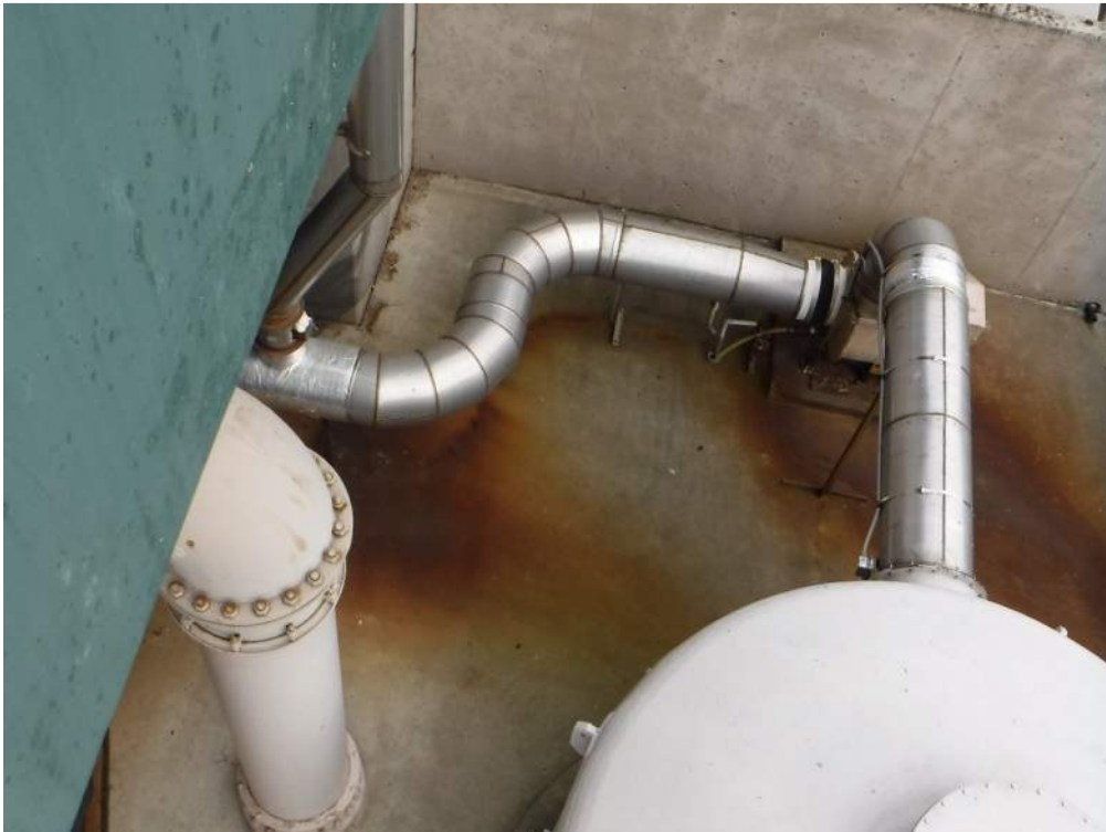
Photo 42. Rust staining on concrete floor under stainless steel odor control duct with penetrations caused by internal corrosion.
