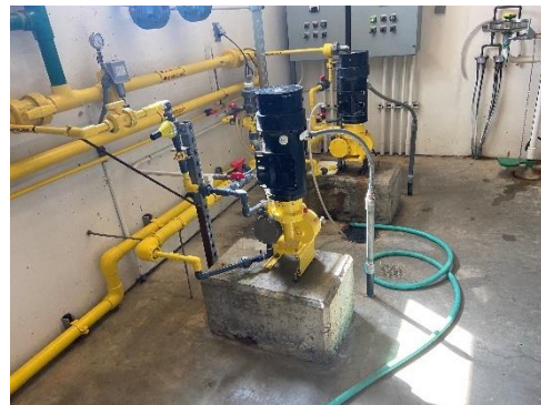
WWTF Chlorine Pumping Room
