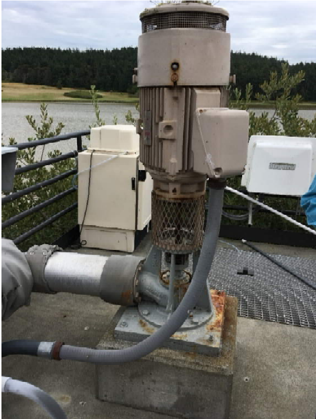
Photo 16: W3 pump and Effluent Sampler
