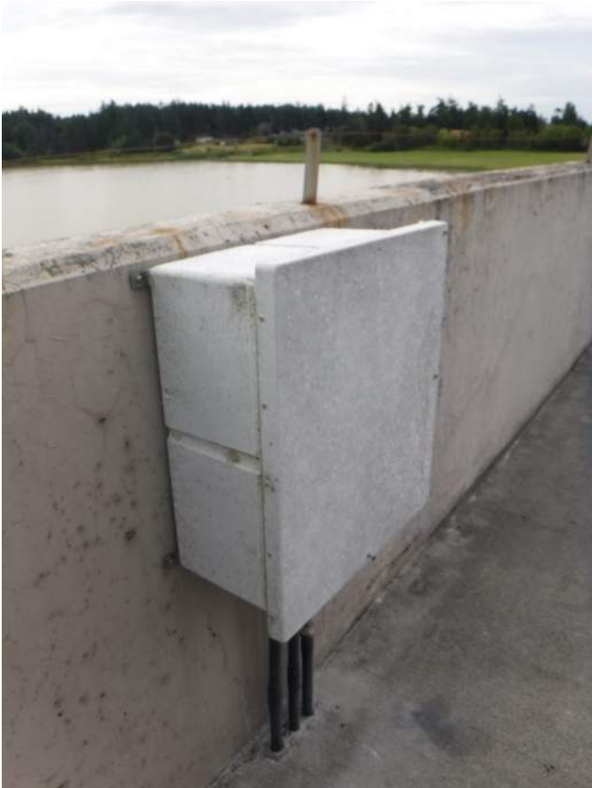
Photo 41. Fiberglass box housing instrument panel, subject to UV deterioration (east side of headworks).
