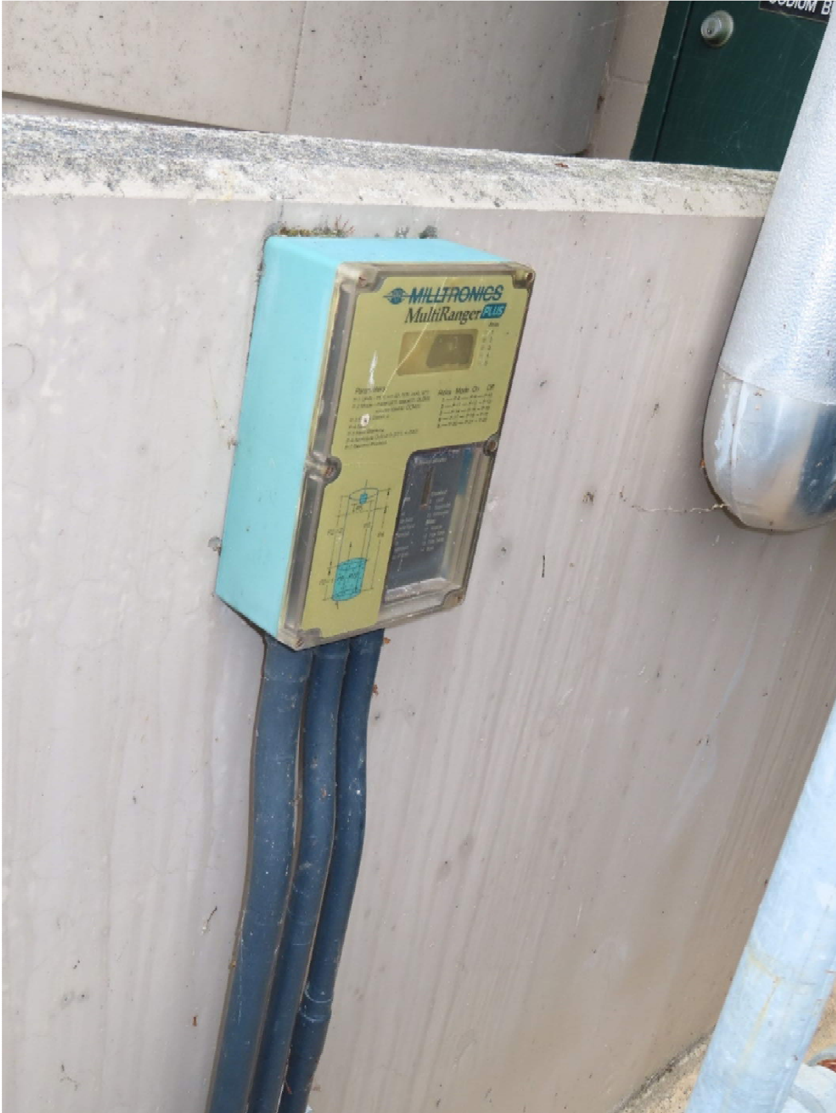
Photo 32. Abandoned the Milltronics transmitter
