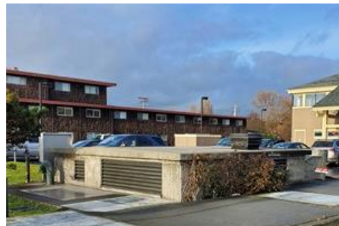
Gaines Street Lift Station
