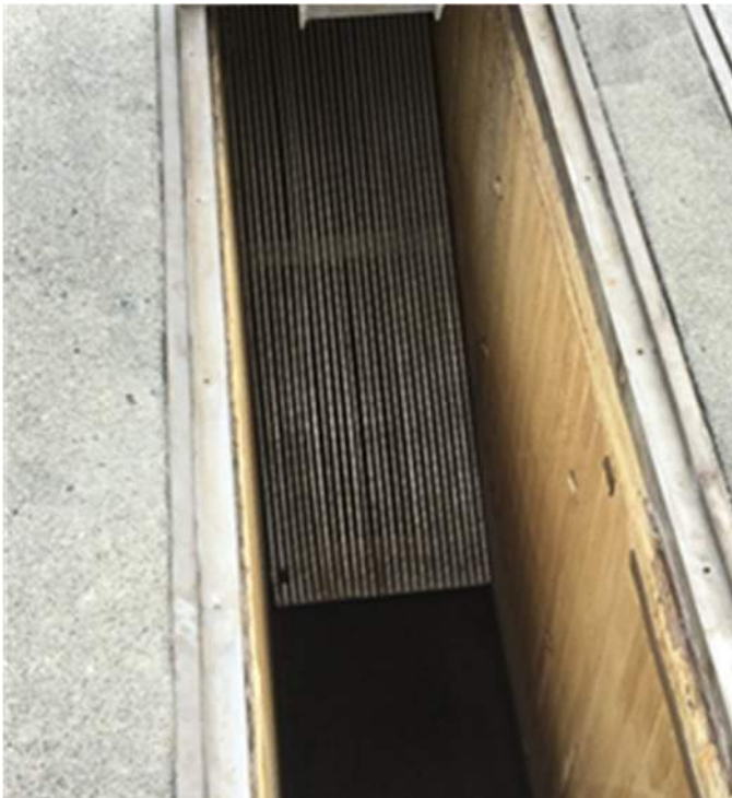
Photo 2: Bar Screen in Channel
