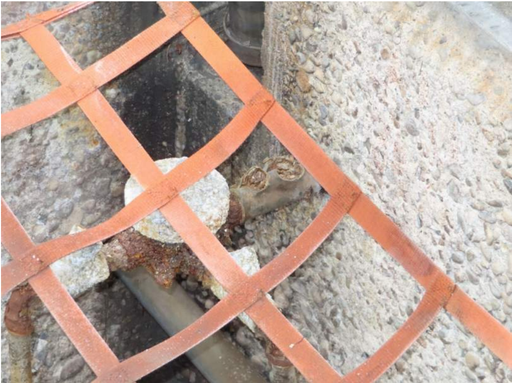
Photo 28. Gas transmitter experiences extreme corrosion
