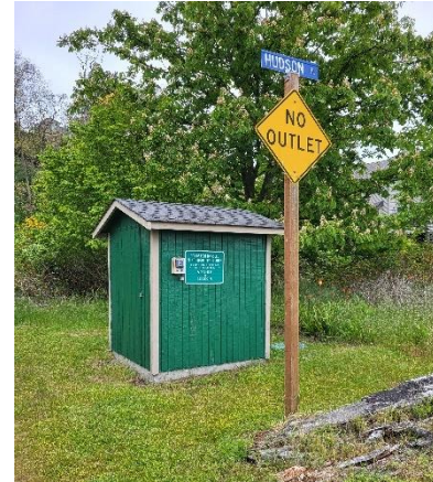
Point Hudson Lift Station
