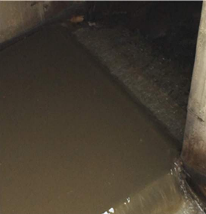
Photo 1: Oxidation Ditch Influent/RAS Splitter Box
