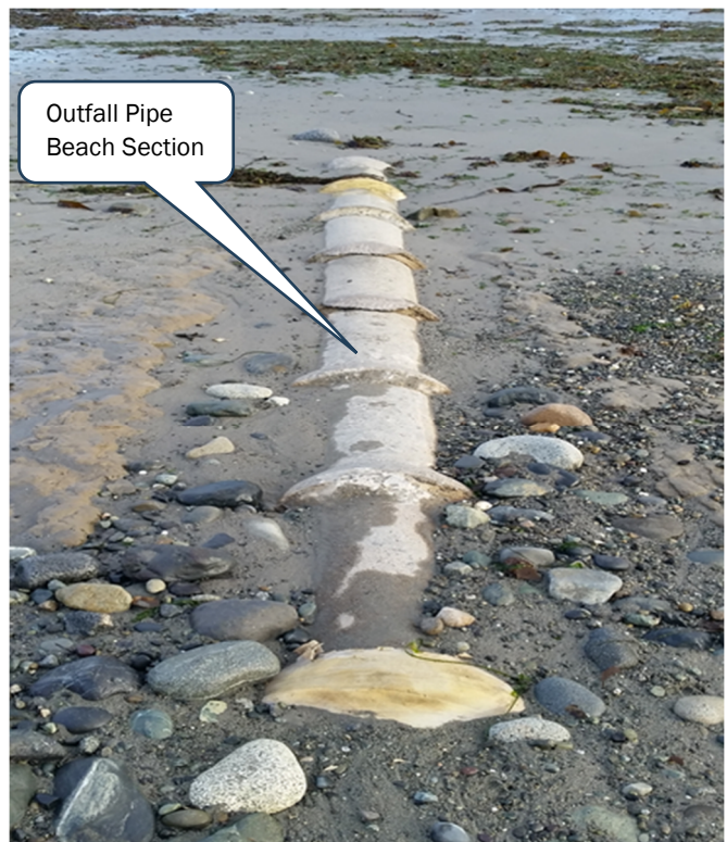
Existing Outfall with Documented History of Leaks from Storm Damage The Outfall Diffuser is Also in Need of Replacing
