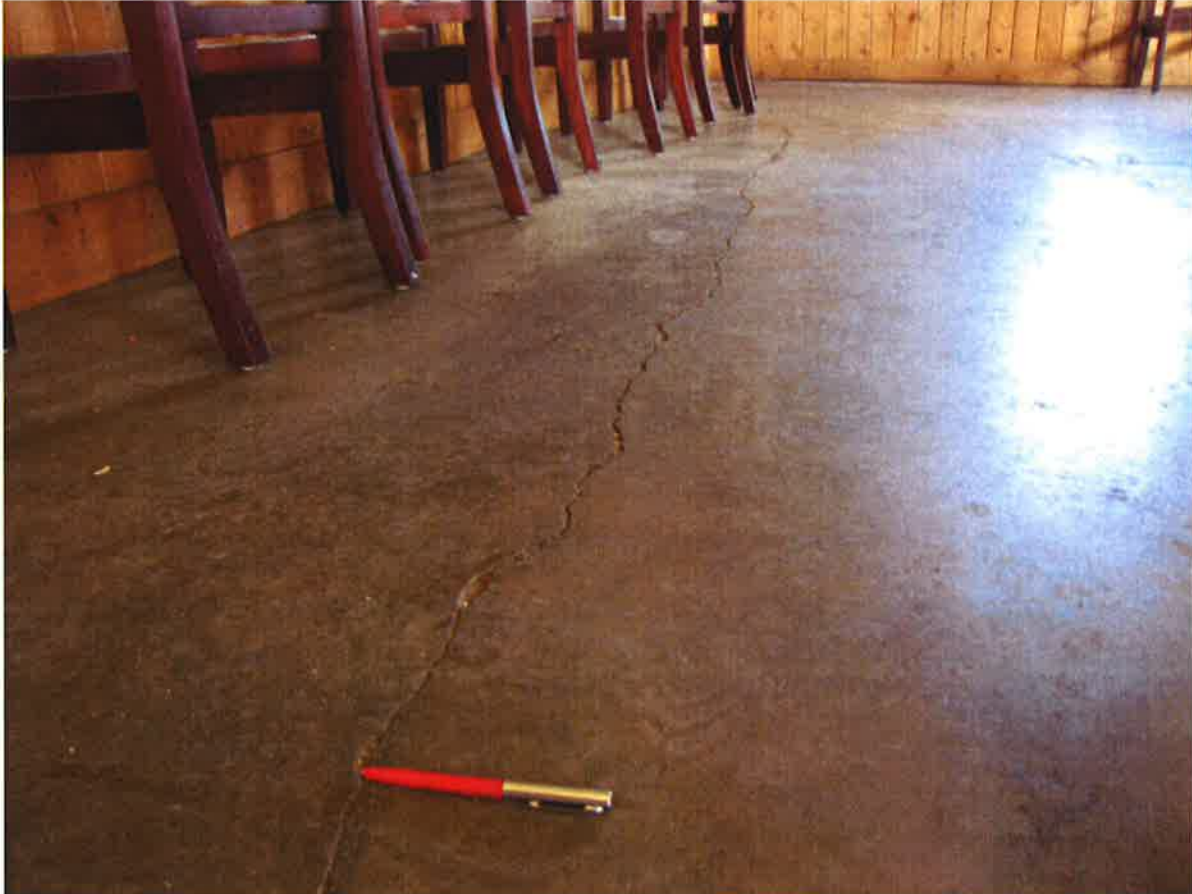
Photo 2: Crack in the brewery's tasting room floor running north south and extending into the pavement to the south, outside the building.
